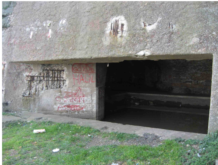
Fig. 2.86 Photograph from Garipçe fortress, third terrace embrasures from the outside, 30 March 2009 (photograph by author).
