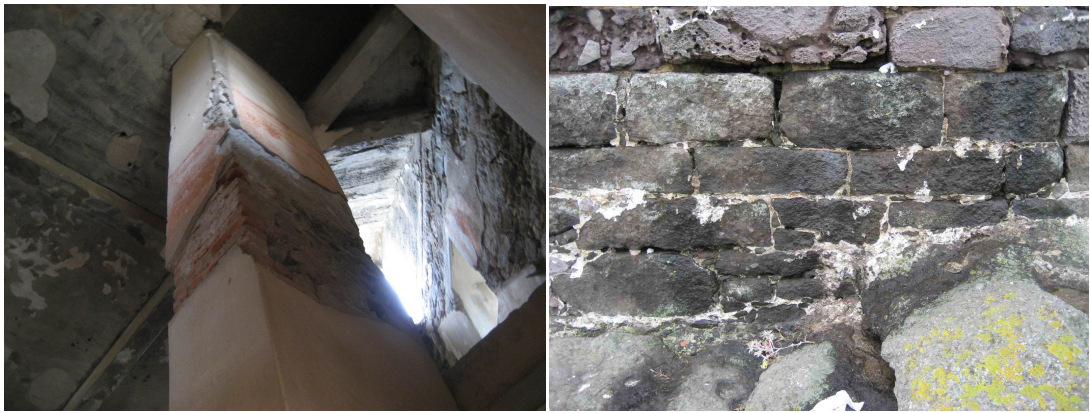
Fig. 4.23a/b Rumelifeneri fortress, interior of north tower on the left with Republican period cement additions and effects of ground water penetration on the right (photographs by author).
