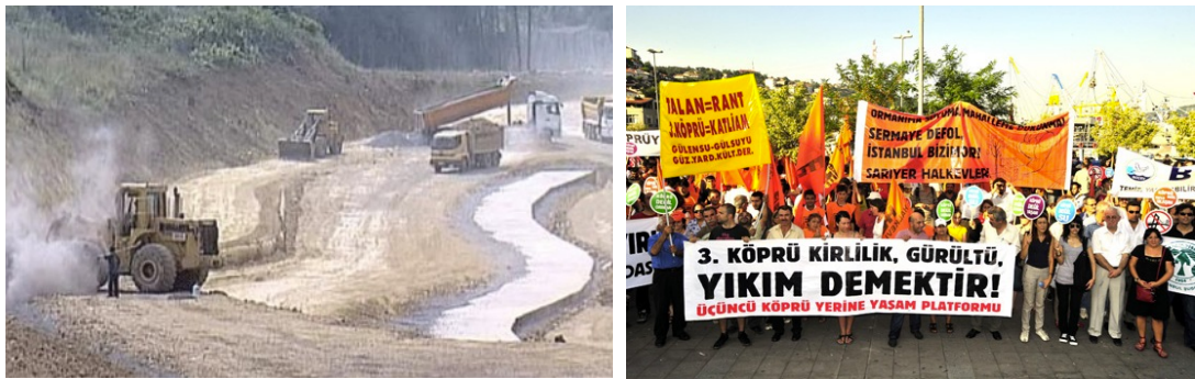
Fig. 4.32 a/b On the left the road constructions ( Radikal 6 July 2009). On the right, protests against the 3 rd bridge (Mimdap.org)
