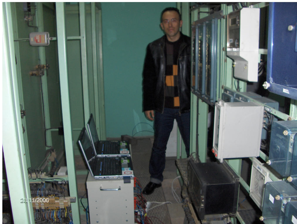
Figure A.3 A photo from on-line power quality analysis in Alaçatı Substation.
