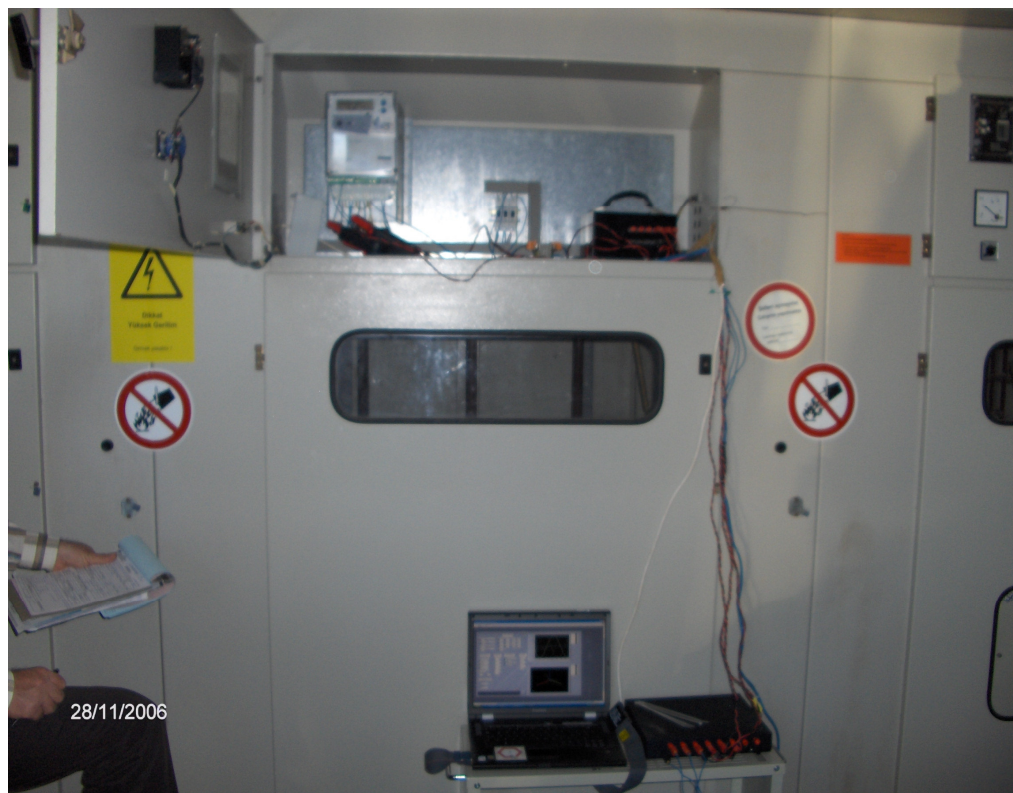
Figure A.2 A photo from on-line power quality analysis.
