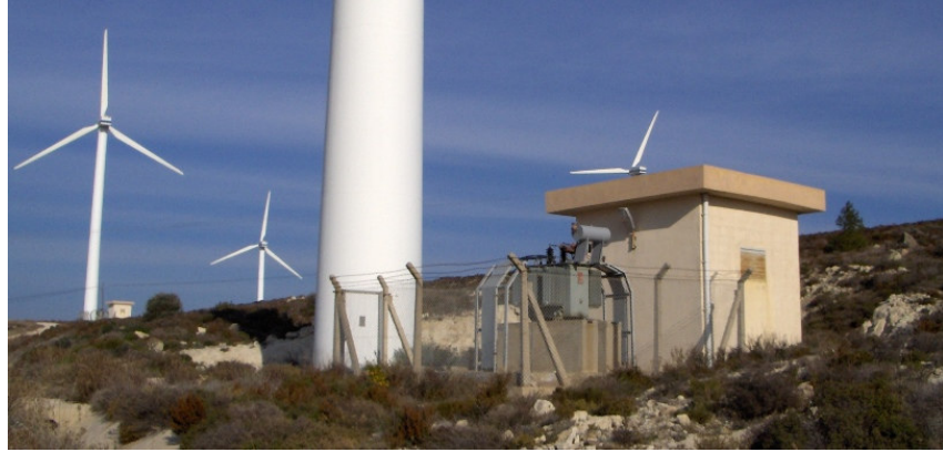
Figure 4.2 Wind turbine 0.69/34.5 kV star-delta connected transformer in wind farm.
