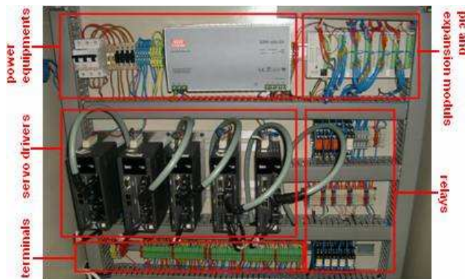
Figure 3.26 Main panel general view
