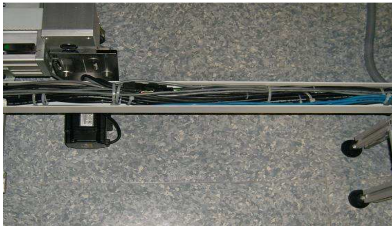
Figure 3.19 Cable channel between main panel and remote equipments
