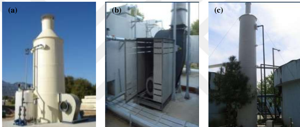
Figure 2.13 Wet scrubbers from different sectors (a), (b) from wastewater treatment plants, (c) alcohol production
