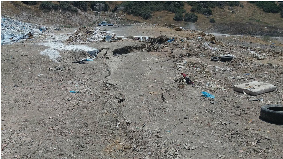
Figure 5.10 The tension cracks and fractures which occurred resulting from landslide event in the Harmandalı waste disposal site (Personal archive, 2018)
