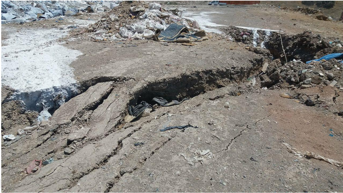
Figure 5.9 The tension cracks and fractures which occurred resulting from landslide event in the Harmandalı waste disposal site (Personal archive, 2018)
