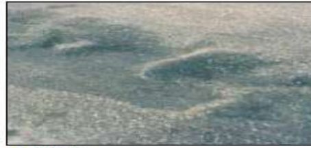
FIGURE 35 Distress Type ACP 10—Shoving in Pavement Surface
