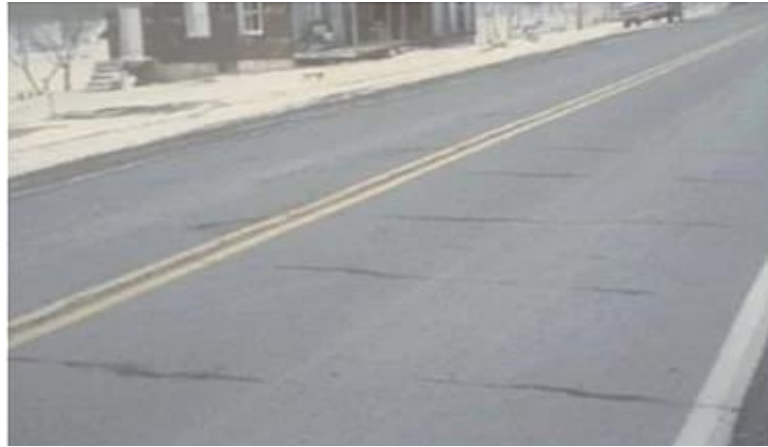
Figure 3.13. Transverse cracking in asphalt flexible pavement [55].
