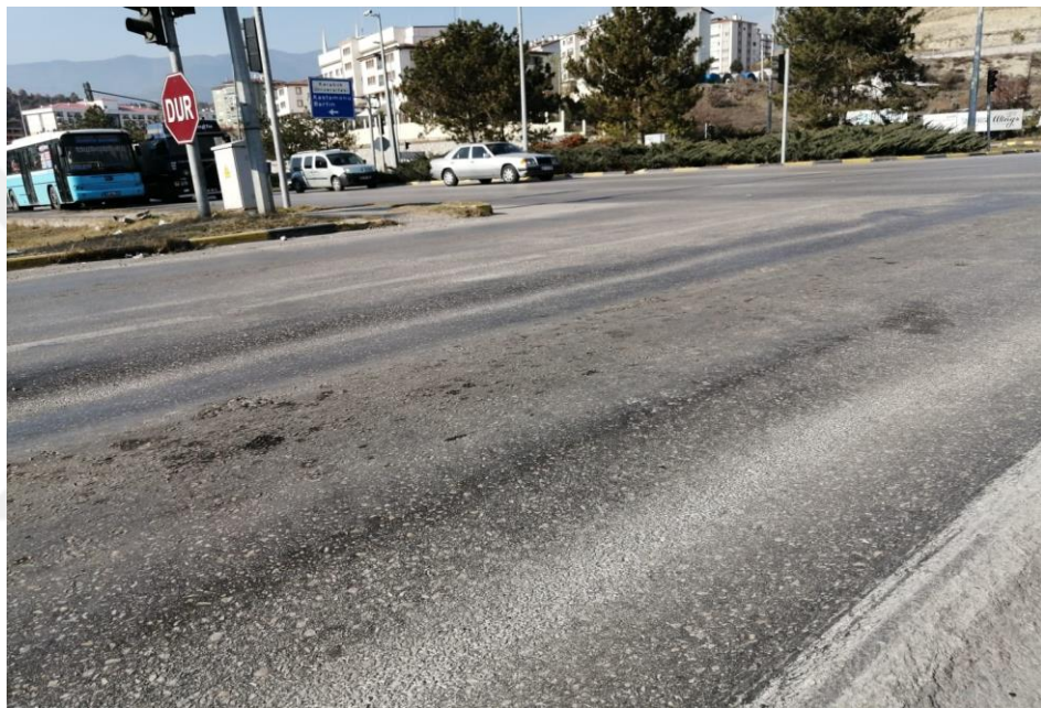
Figure 5.1. Asphalt rutting and deformations in Karabük – Turkey.
