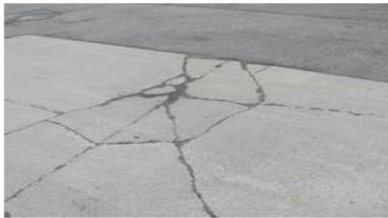
Figure 3.26. Punch-out failures in rigid pavements [60].
