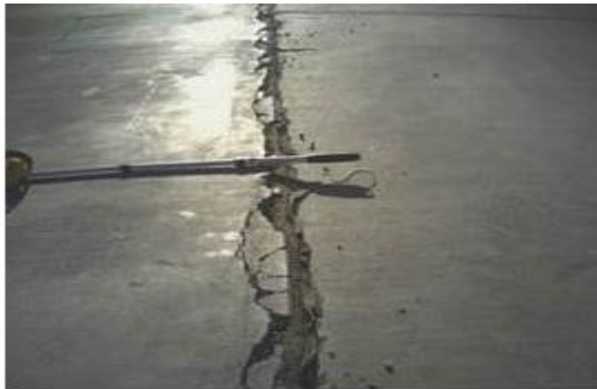
Figure 3.21. Faulting with difference in elevations at rigid pavement [60].
