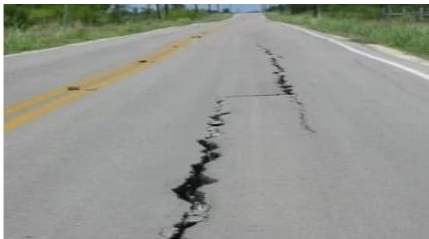
Figure 3.12. Longitudinal cracks in asphalt flexible pavement [55].
