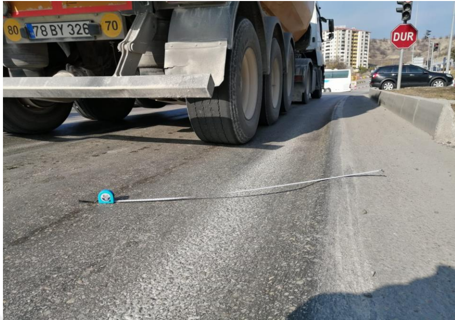
Figure 5.2. The rutting and deformation of asphalt in Karabük - Turkey.
