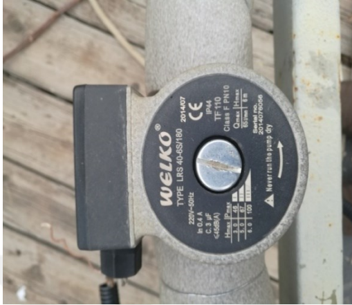
Figure 2. 15 Adjustment water pump
