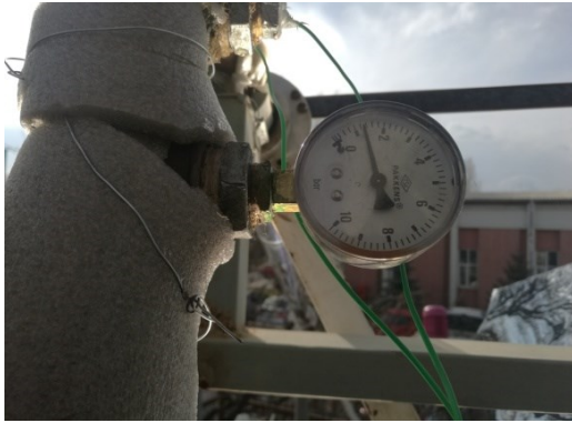
Figure 2.19 Pressure gauge & thermo cable
