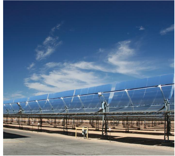
Figure 1. 18 Collectors Field of PTC plant.
