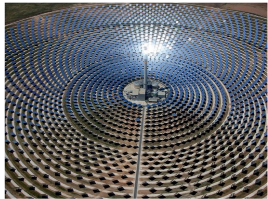
Figure 1. 22 Solar field of tower plant.
