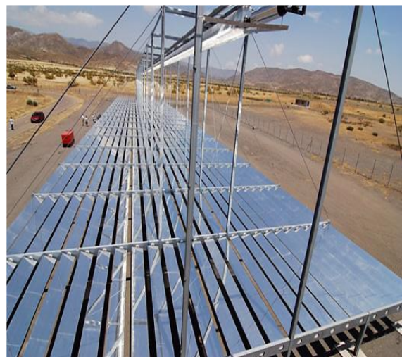
Figure 1. 20 LFCS platform solar reflector.
