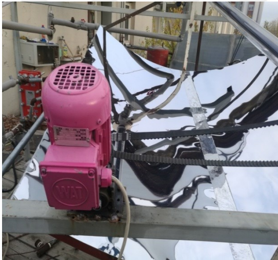
Figure 2.21 Collector driver motor
