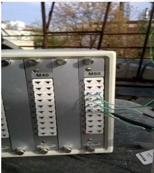
Figure 2. 17 Thermo cable temperature reader
