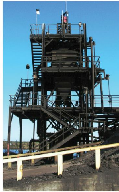
CrossFlow Separator installation for the recovery of heavy mineral.
