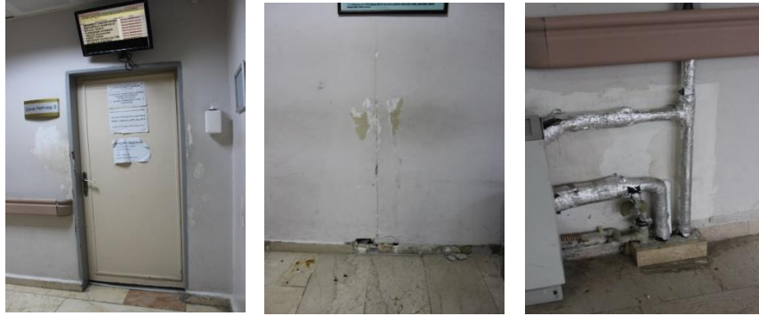
Figure 47. Example of the condition of the materials used in the polyclinic.
