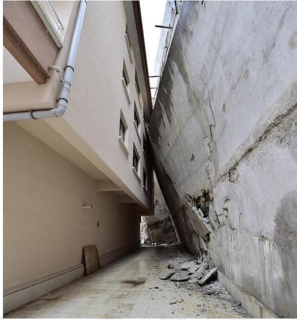
Figure 3.3. Landslide event occurred in Cengizhan Neighborhood on Nov 1, 2014 [76].
