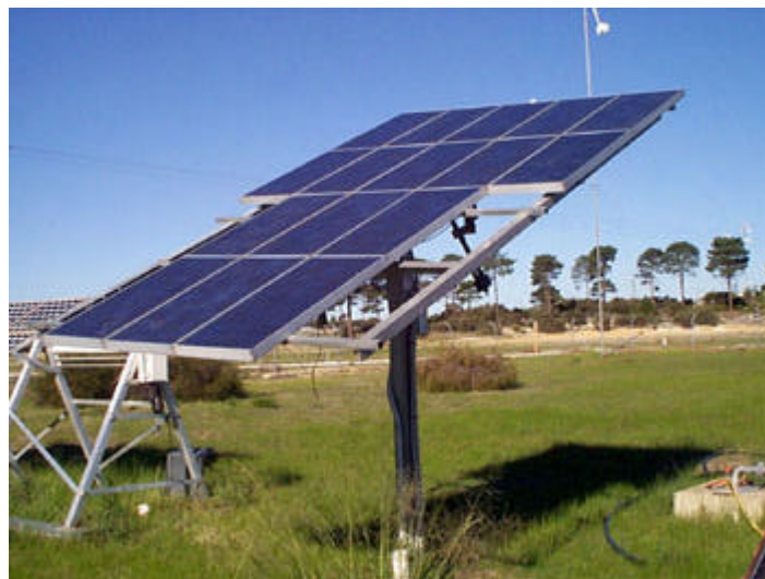
Figure 4.2 Tracked PV Array
