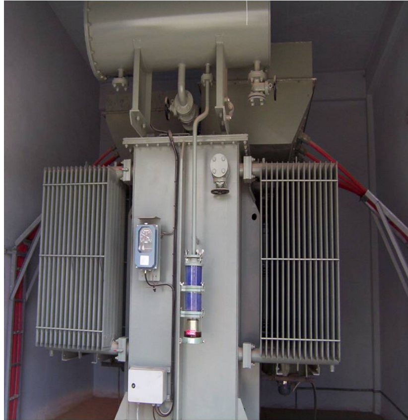
Figure 7.8 The Alstom transformers in SANKO DEPC
