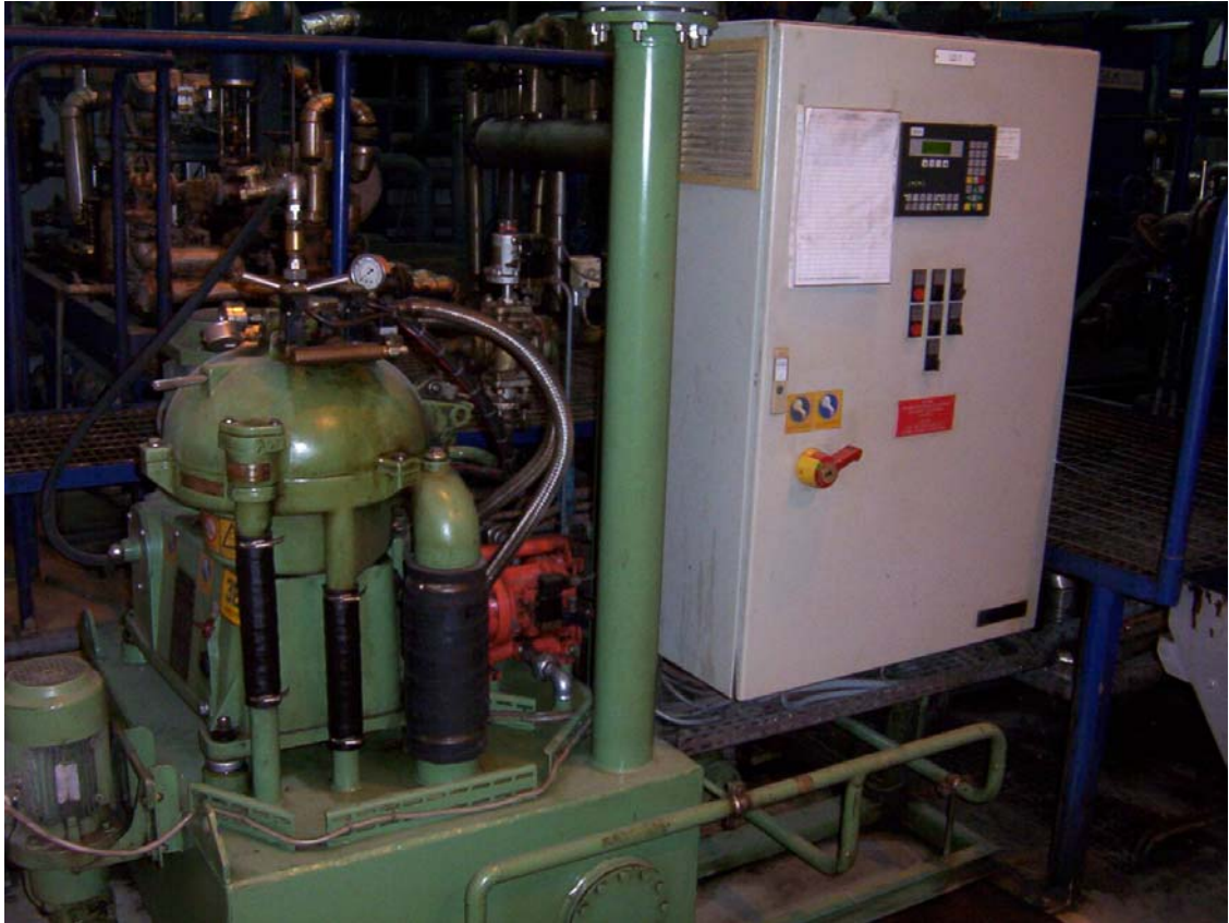
Figure 7.14 Lubrication oil filter system in SANKO DEPC
