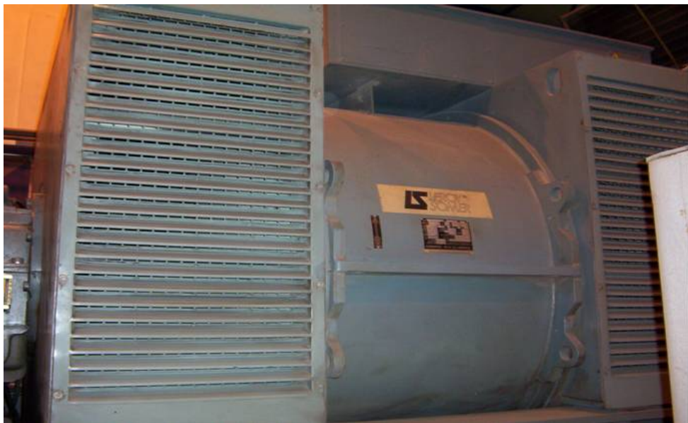
Figure 7.7 The Leroy-Somer generator in SANKO DEPC
