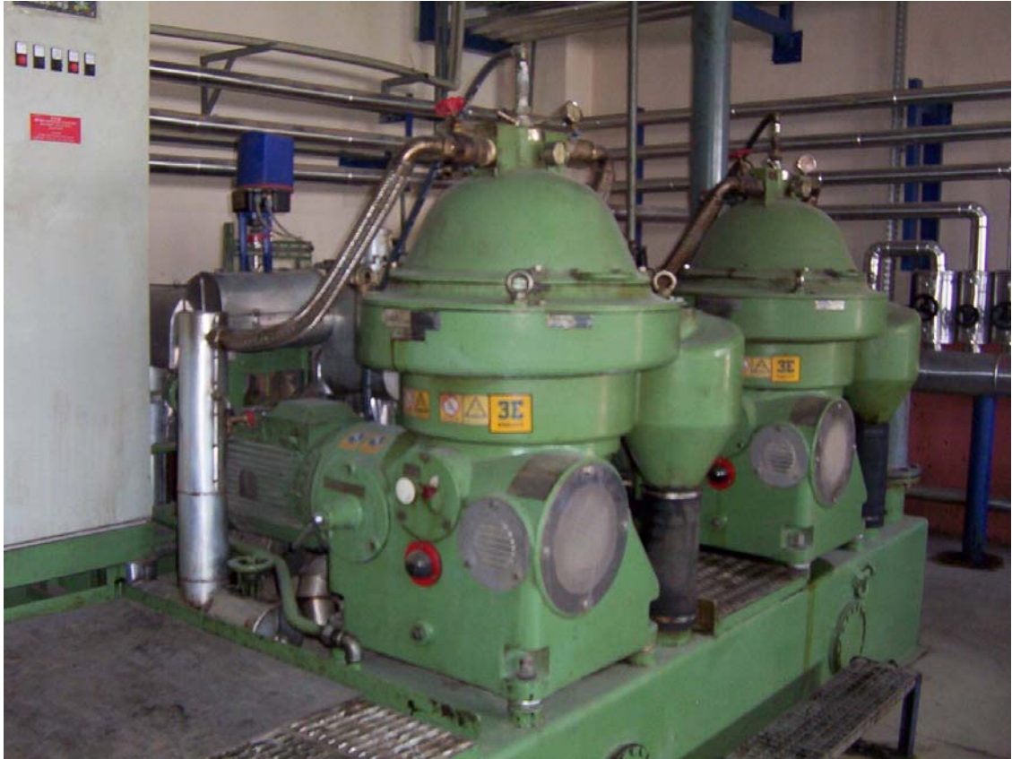
Figure 7.12 The fuel separator of fuel forwarding module in SANKO DEPC
