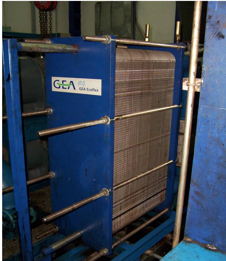
Figure 7.13 Lubrication oil cooler (LOC) in SANKO DEPC
