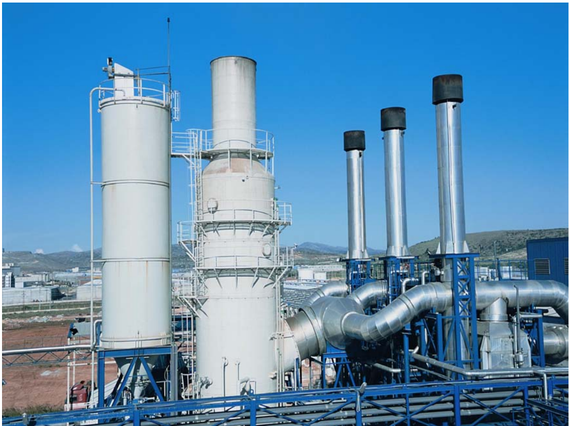
Figure 7.18 Exhaust gas treatment unit in SANKO DEPC
