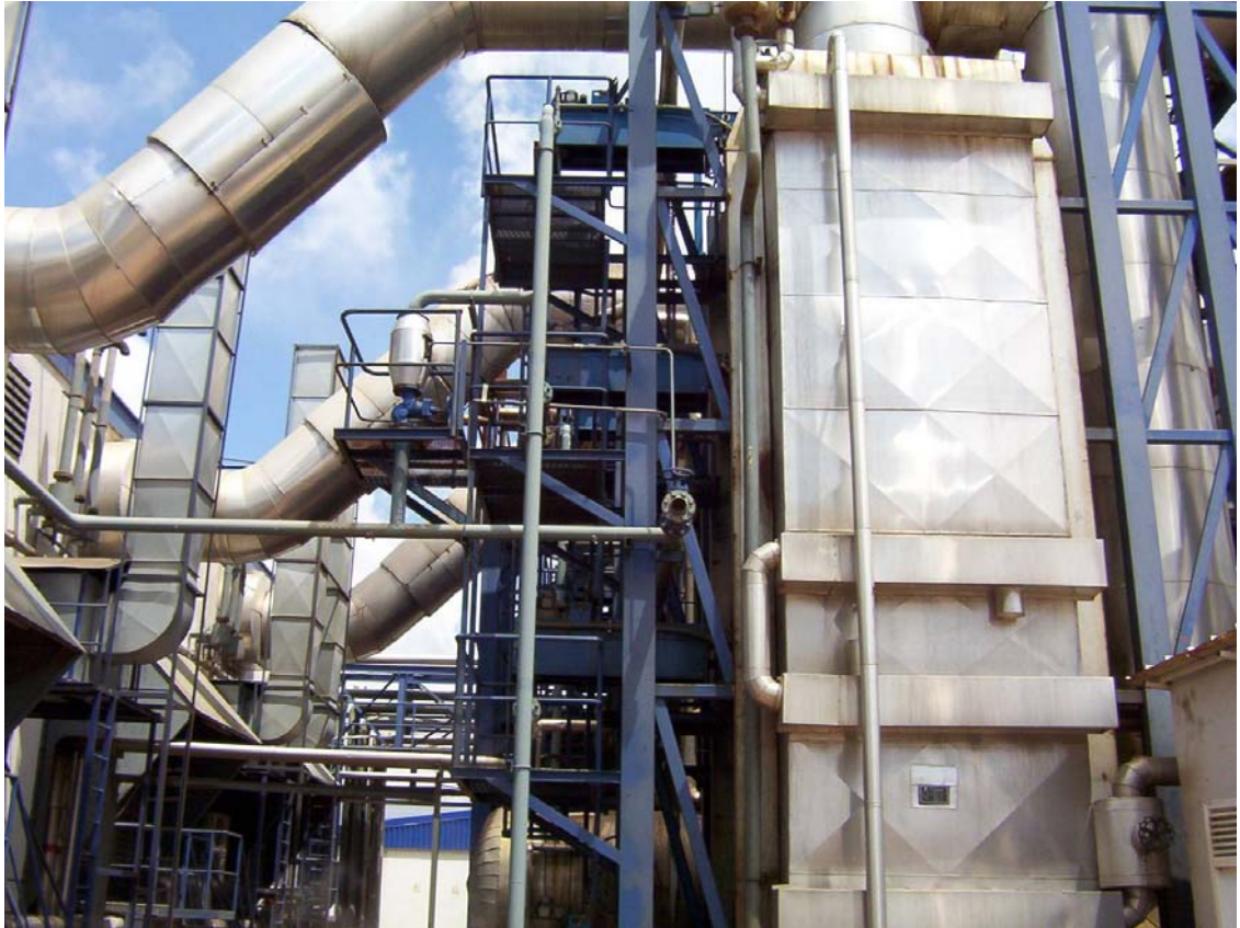
Figure 7.17 Waste heat recovery boiler unit in SANKO DEPC
