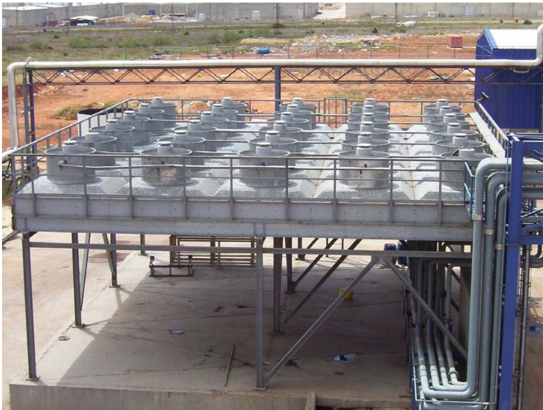
Figure 7.16 Air – water radiator units in SANKO DEPC
