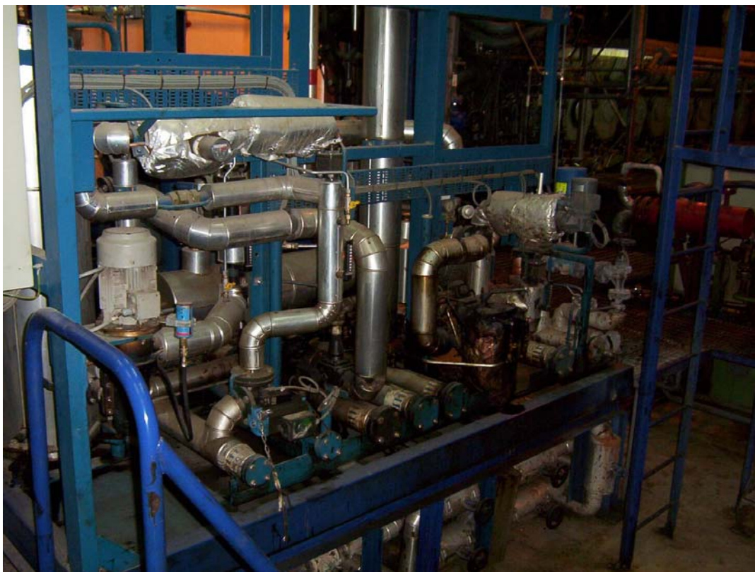
Figure 7.11 The fuel forwarding module (FFM) in SANKO DEPC
