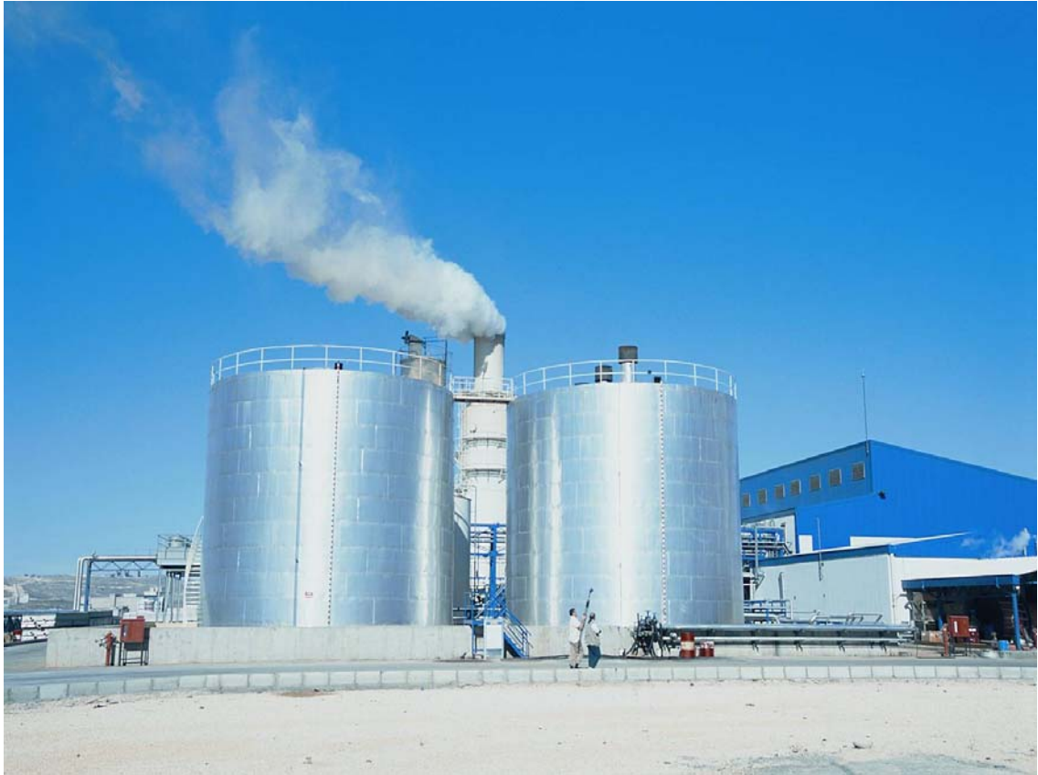
Figure 7.3 The views of the HFO and LFO day tanks in Sanko DEPC
