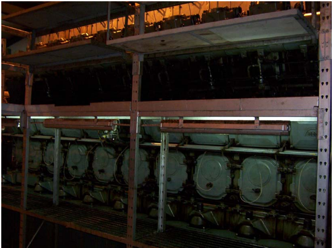
Figure 7.6 The side view of M.A.N Engine 18 V 32/40 in SANKO DEPC Plant
