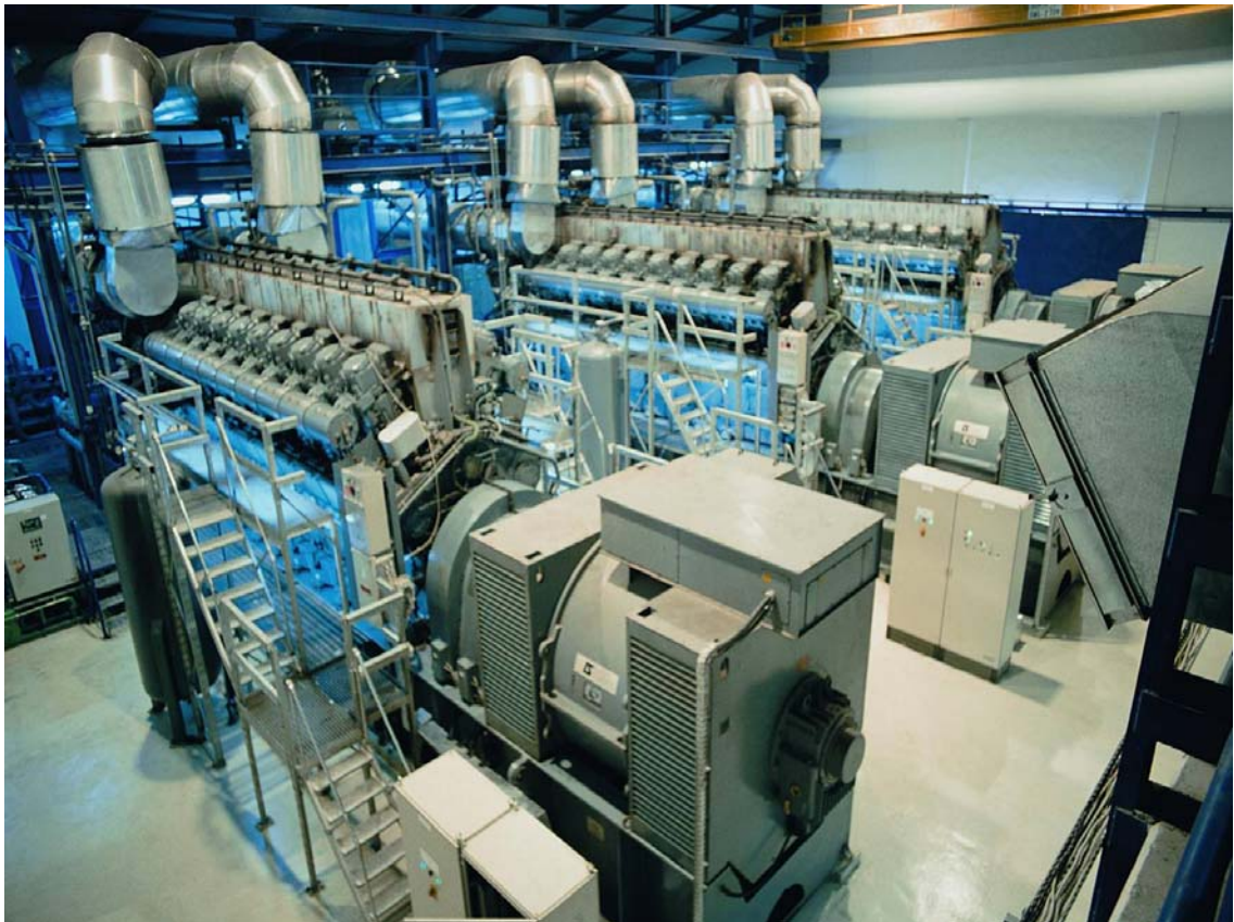
Figure 7.2 The diesel engine actuated generator sets in SANKO DEPC
