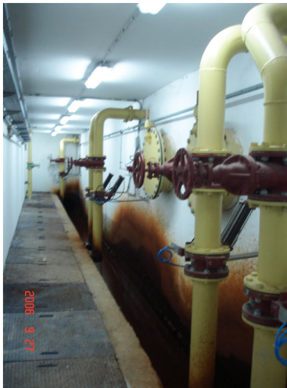
Figure 2.12 Sludge Filter Rooms.
