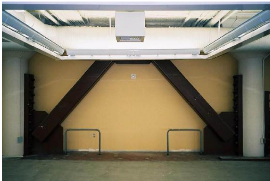
Figure 2.4 An example of inverted V type steel braces application for seismic retrofit (Coşkun, 2010)
