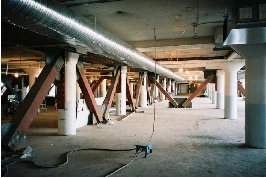
Figure 2.5 An example of V type steel braces application for seismic retrofit (Coşkun, 2010)
