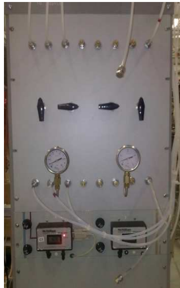
Figure 3.15: Cooling system rack panel.
