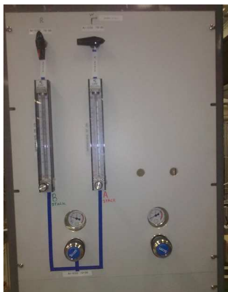
Figure 3.13: Active gas system rack panel.
