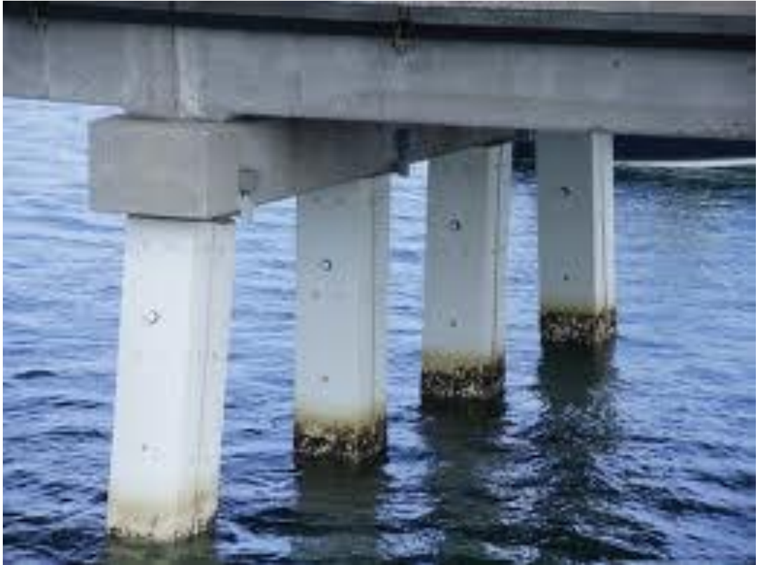
Figure 2.5 Bridge pier under severe chloride attack ( http://www.compositesworld.com/articles/composite-vs-corrosion-battling-for-marketshare )
