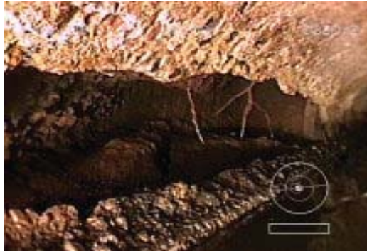
Figure 2.4 Eroded concrete in sewer pipe [25].
