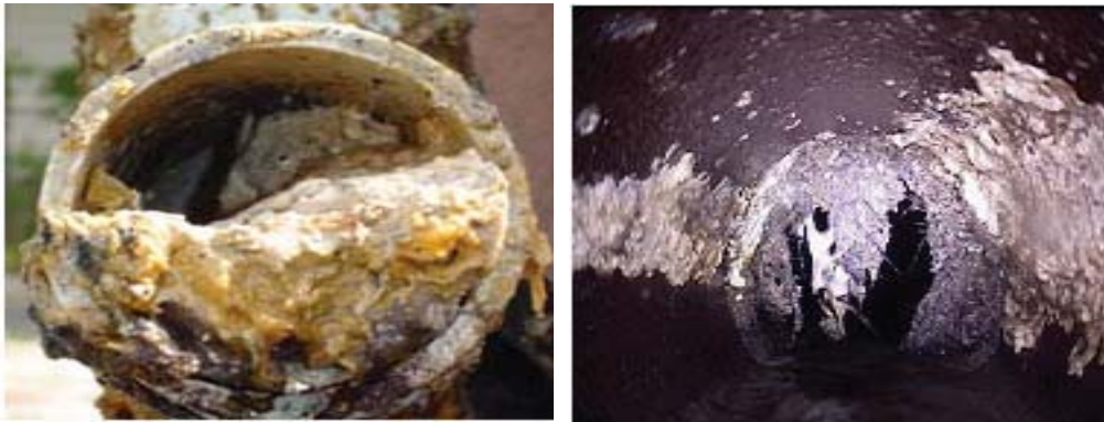
Figure 2.3 Grease buildups in sewer pipe [7].
