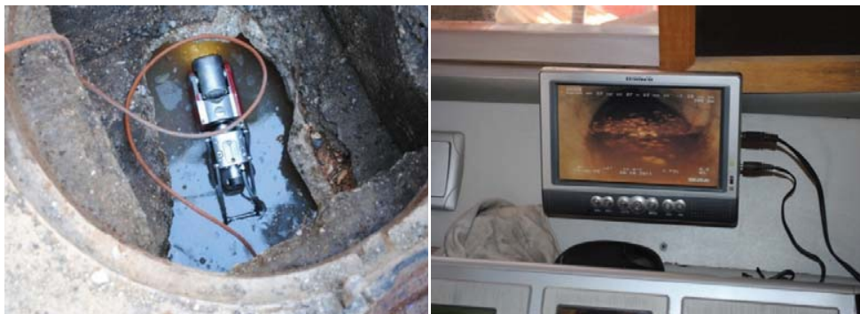
Figure 3.19 Robot about to move. Figure 3.20 Shows pipe image from inside.
