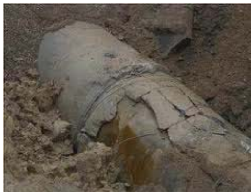
Figure 2.6 Indicates corrosion of a concrete pipe [28].
