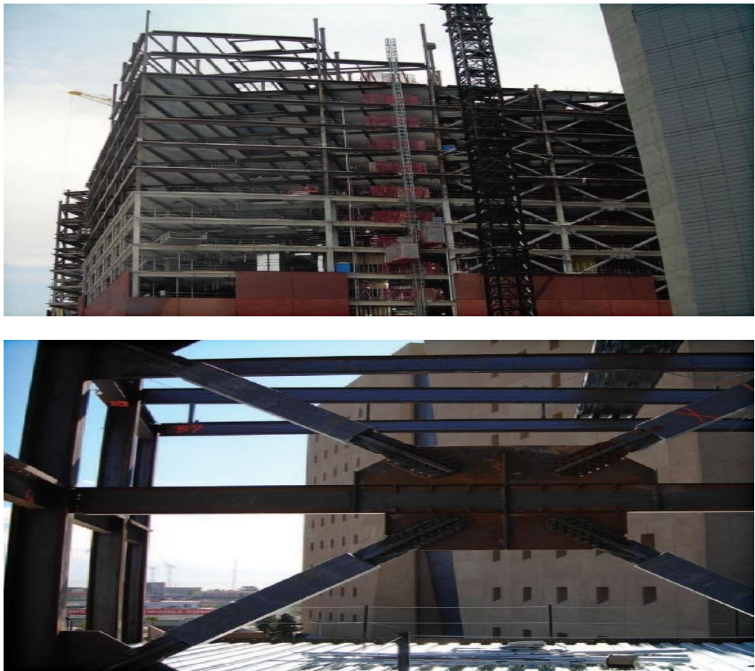
Figure 2.22 Use of BRB in world market center III, Las Vegas, Nevada (Corebrace, 2002)
