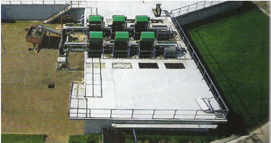
Figure 7.2: Coarse and fine screens of the GASKI WWTP
