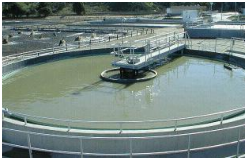
Figure 7.4: Primary sedimentation tanks of the GASKI WWTP
