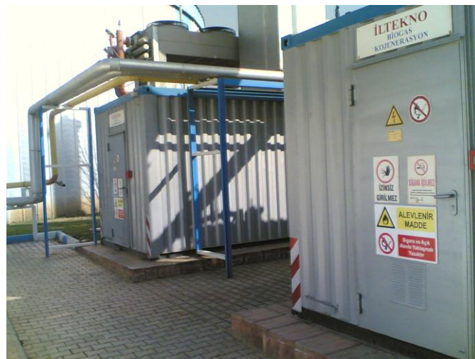
Figure 7.11: GASKI Biogas Engine Powered Cogeneration System
