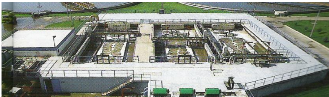
Figure 7.3: Grit and grease removal tanks of the GASKI WWTP
