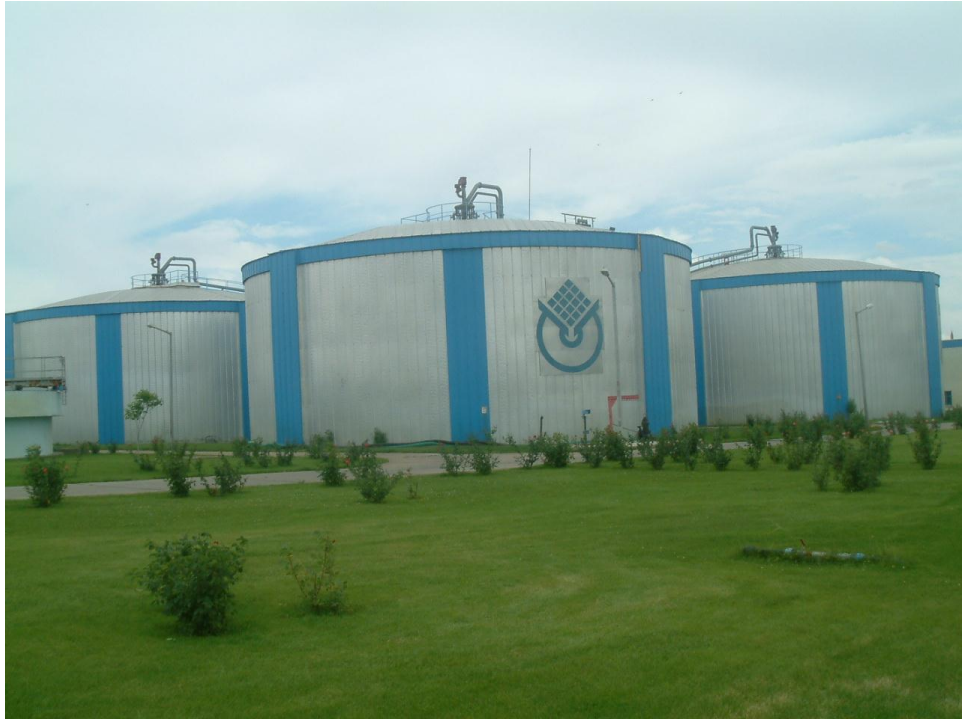
Figure 7.8: Anaerobic digestion tanks of the GASKI WWTP
