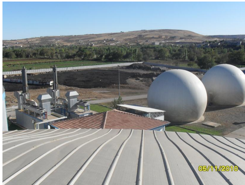
Figure 7.9: The views of the biogas store tanks in GASKI WWTP
