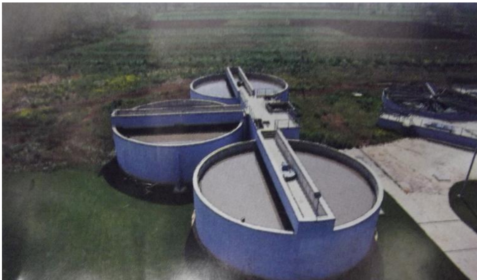
Figure 7.7: Thickening tanks of the GASKI WWTP
