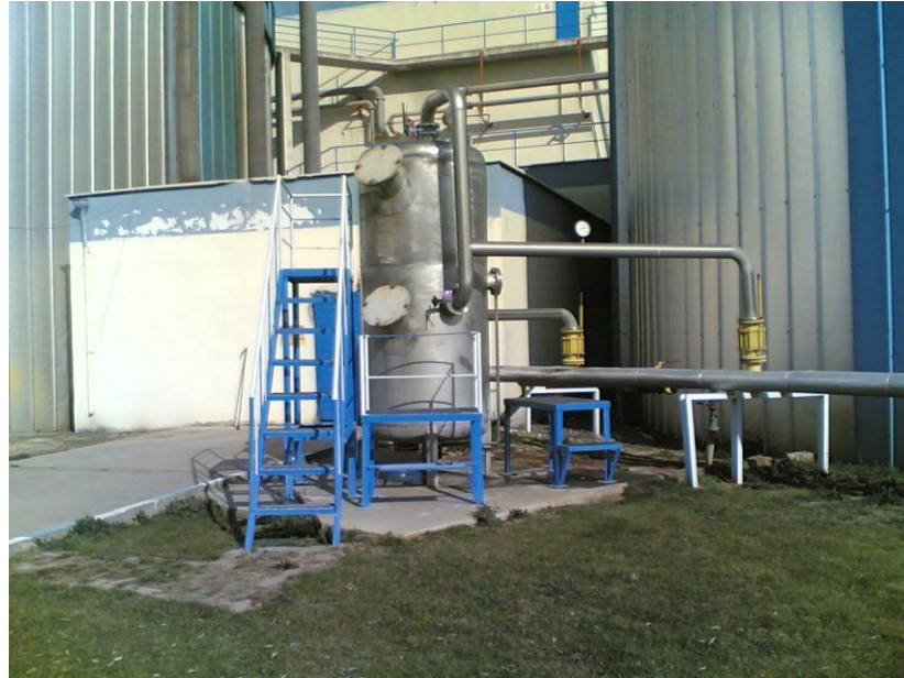
Figure 7.10: A view of the DeSO x unit in GASKI WWTP
