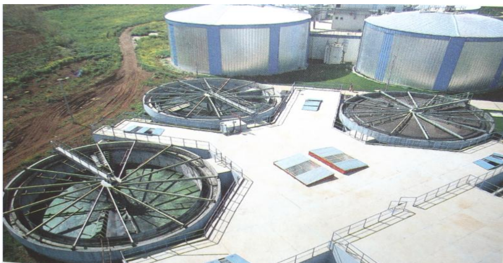
Figure 7.6: Flotation tanks of the GASKI WWTP
