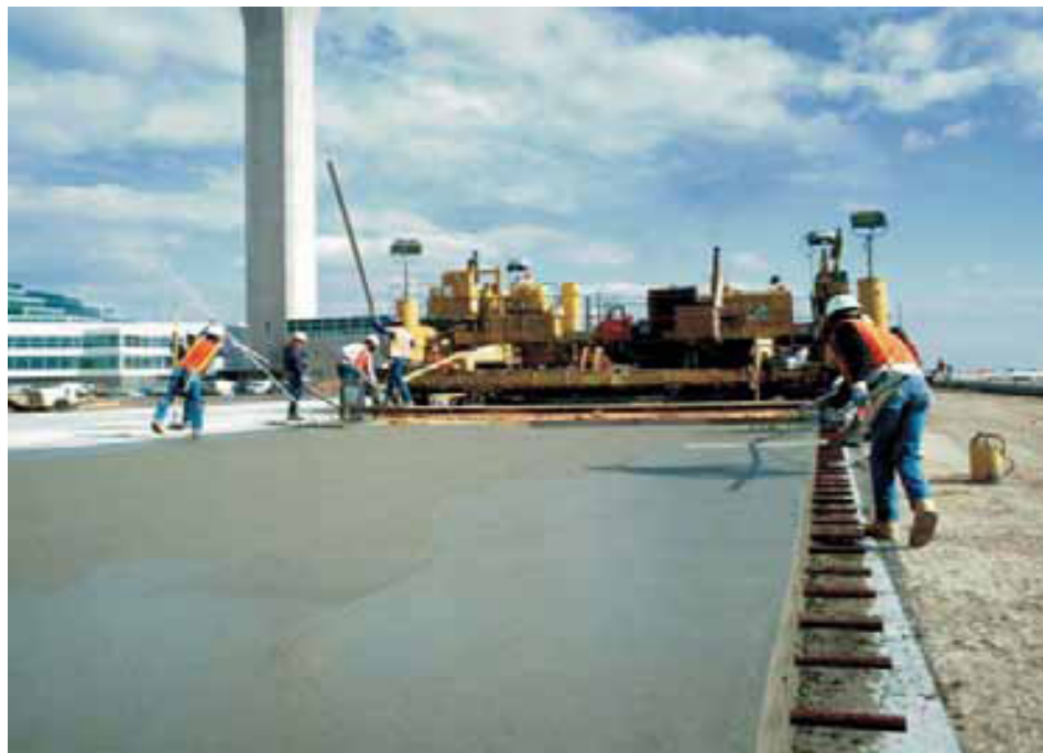
Figure 2.3 Application of high early strength concrete for airport aprons and taxiway replacement at Philadelphia International Airport, Pennsylvania
