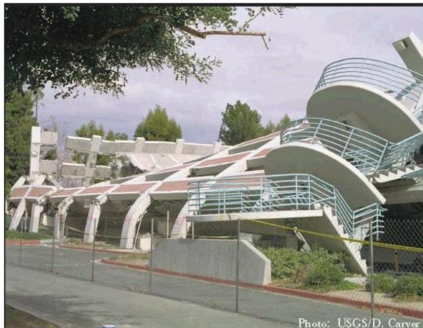
Figure 2.1 1994 Northridge parking structure (California) ( www.vibrationdata.com/earthquakes/northridge.htm )
