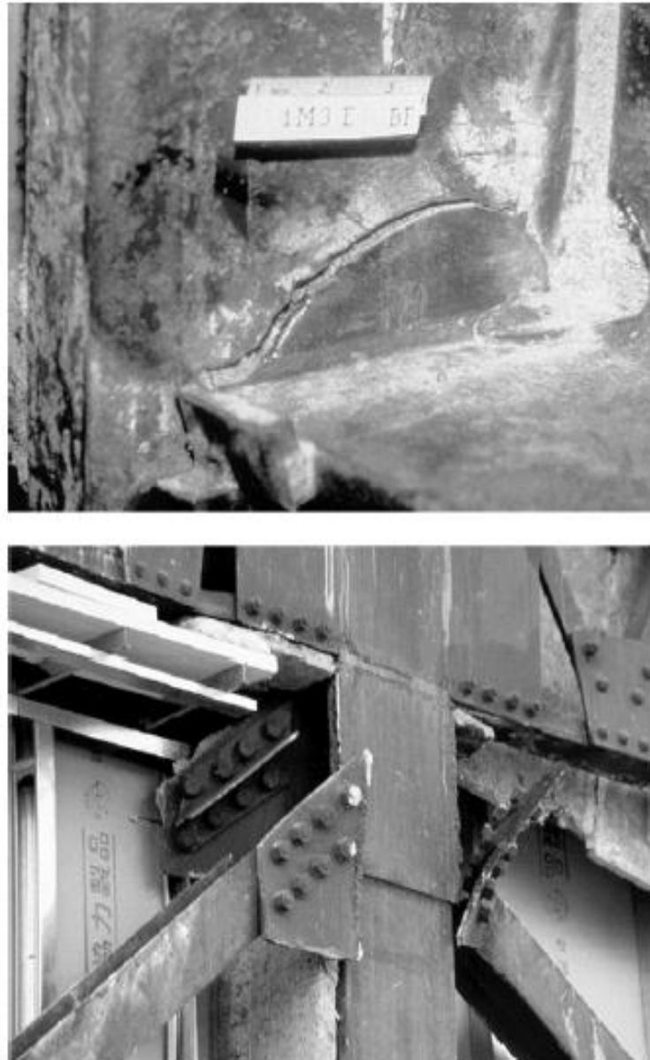
Figure 2.12 Fracture in beam-to-column connections in the Northridge earthquake (top) and web tear-out in bolted brace-to-column connections during the 1995 Kobe earthquake (bottom) (Di Sarno and Elnashai, 2009)
