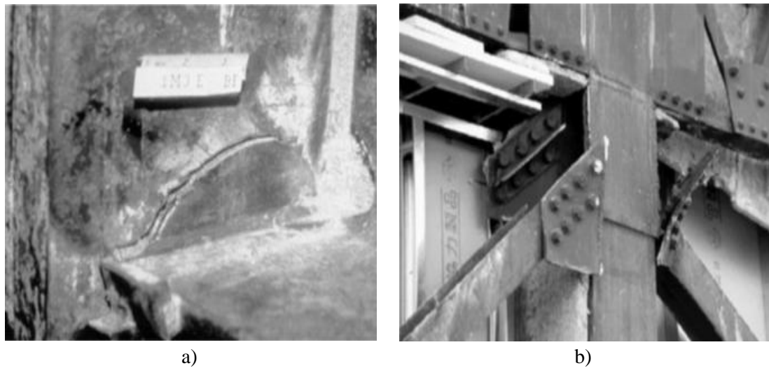
Figure 2.3 View of a) Rupture in column-to-beam connections in the Northridge earthquake and b) web tear-out in bolted column-to-brace connections during the 1995 Kobe earthquake (Di Sarno and Elnashai, 2009)
