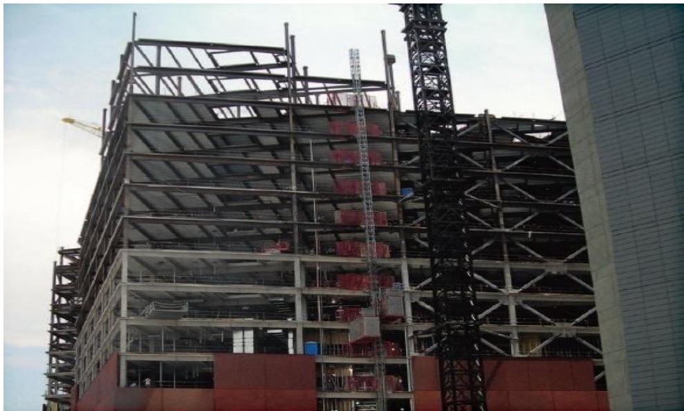
Figure 2.38 Use of BRB in world market center III, Las Vegas, Nevada (Corebrace, 2002)
