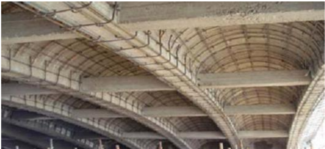
Figure 2.1 General view of placing the steel bars in arch rings (Naser and Zonglin, 2011)
