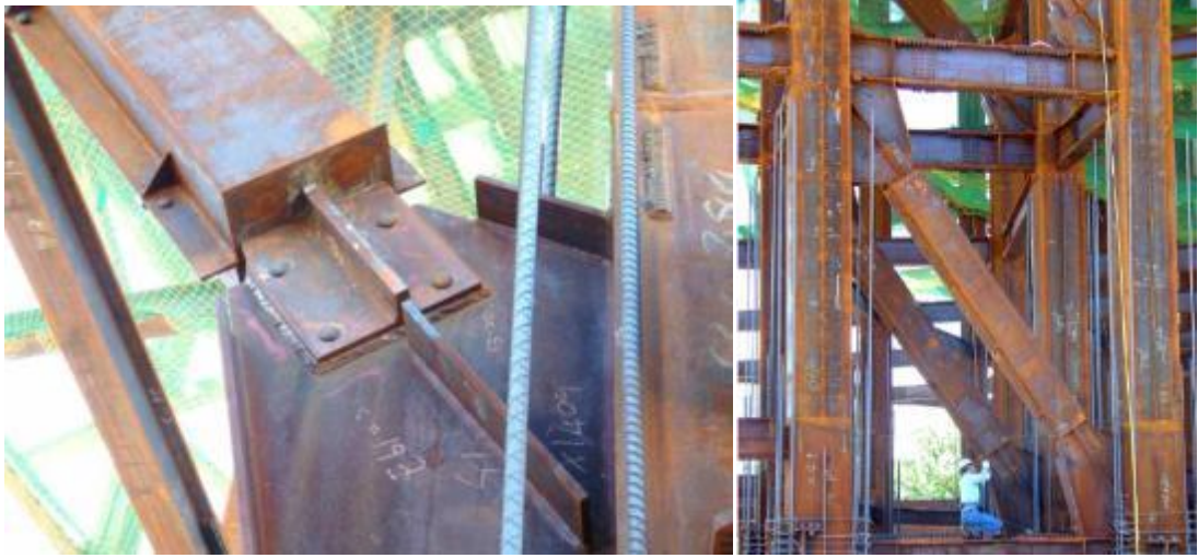
Figure 2.23 Buckling restrained braced frame detail of Tzu-Chi TV Station (in Taipei) (Tsai et al., 2004)
