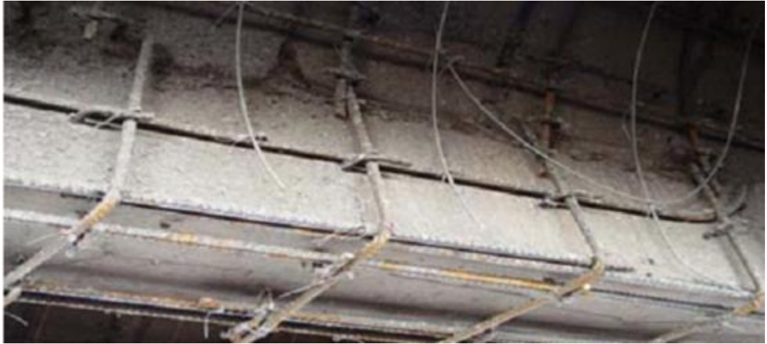
Figure 2.2 Close view of arrangement of steel bars in arch rib (Naser and Zonglin, 2011)
