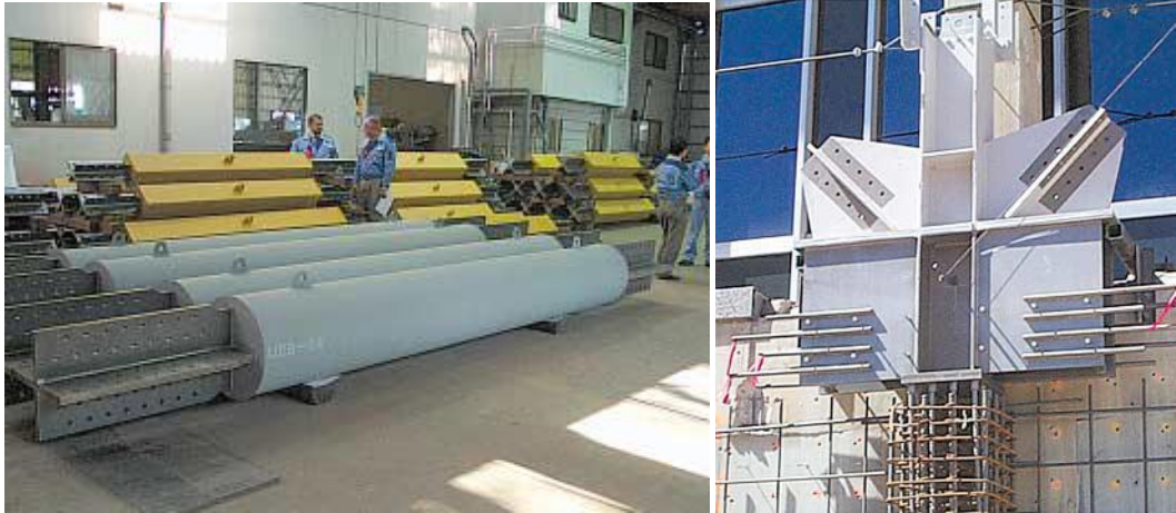
Figure 2.27 Unbonded braces at fabrication plant, Chino, Japan and views of shear transfer assembly as well as brace connection during construction (Brown et al., 2001).
