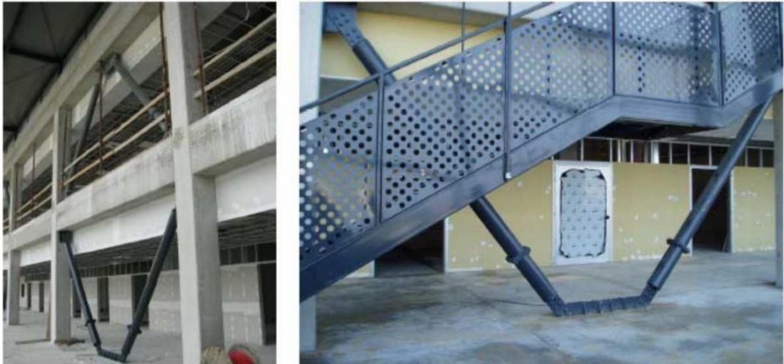
Figure 2.25 Two BRADs installed in the new building of University of Ancona (Eghtesadi, 2010)
