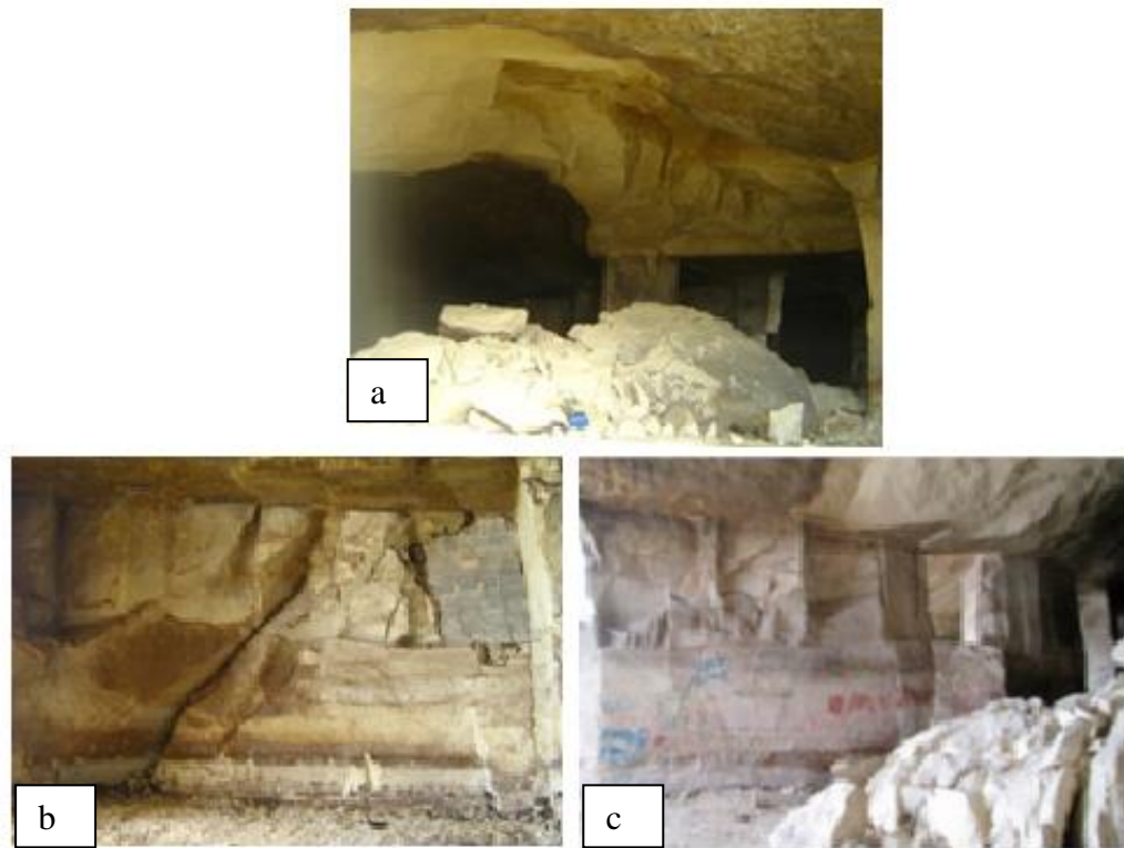
Figure 3.7 Shear failures of rock pillars observed along the section 1-1 of the caves and rock fall in cave no 5
