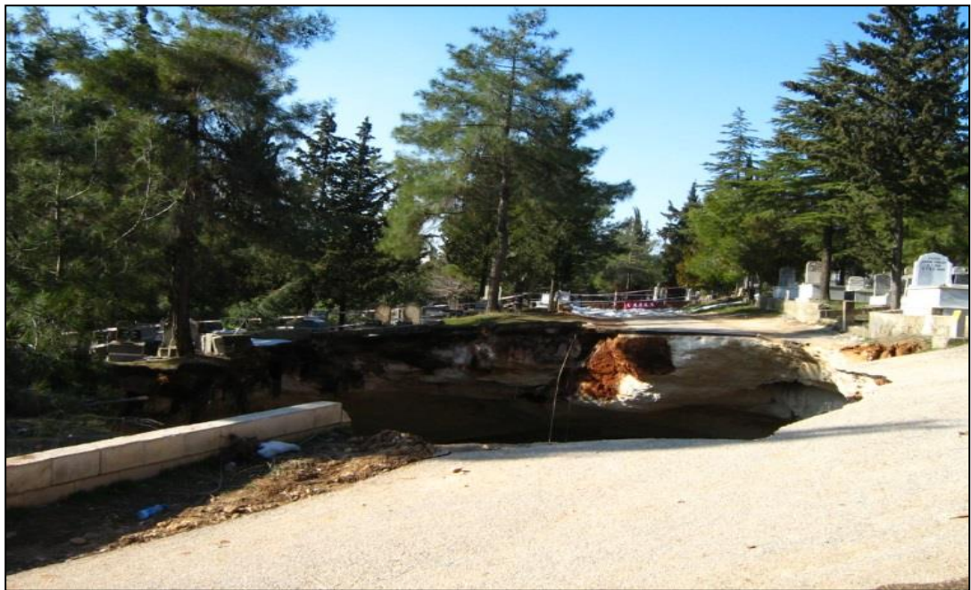
Figure 1.3 Appearance of the sinkhole in Gaziantep Metropolitan Municipality Cemetery
