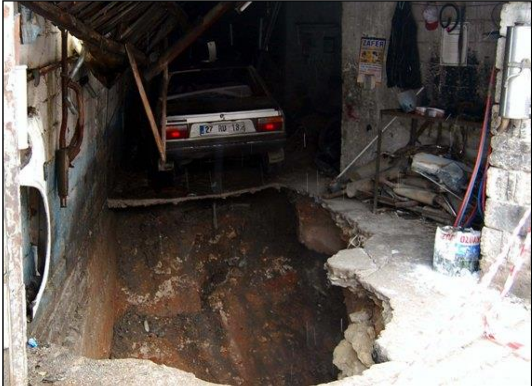
Figure 1.2 Appearance of the collapsed cave in Çamlıca Neighbourhood (Gaziantep Metropolitan Municipality)
