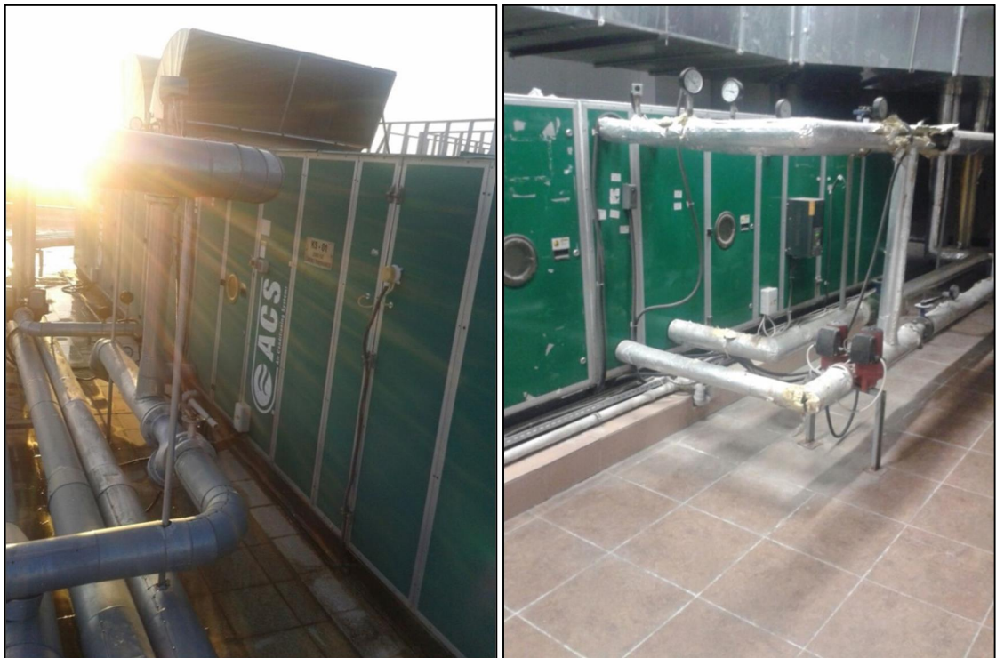
Figure 3.20 Connection of AHU units
