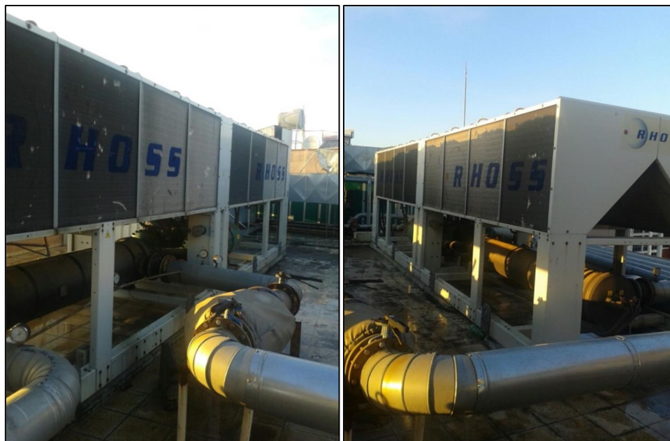
Figure 3.25 Air cooled water chiller
