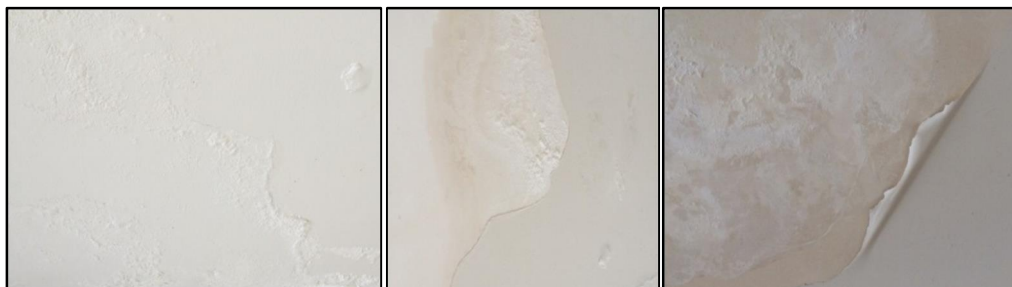
Figure 4.4 Deformed wall due to condensed water
