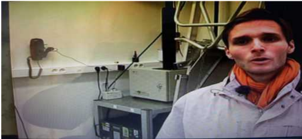
Figure 2.5 Air Pollution Data Collection Cabinet with Piping Connections (2007) [22]
