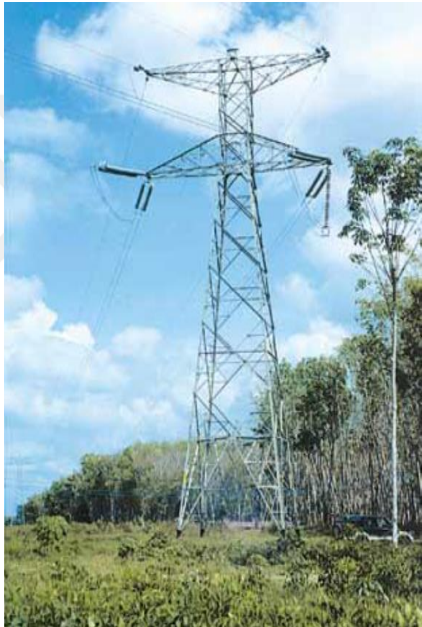
Figure 3.21 DC transmission line tower 300-kV
