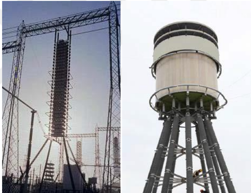
Figure 3.12 Smoothing Reactor and DC-filter with capacitor in HVDC [36].
