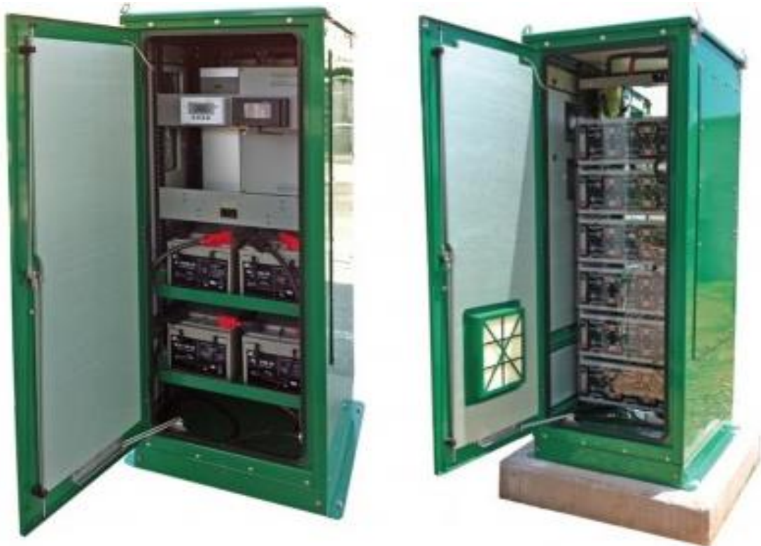
Figure 1.4 Cabinet of Battery Energy Storage System [7]
