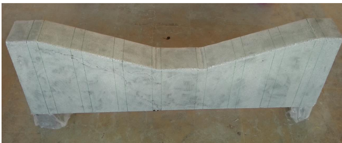
Figure 3.11 Drawing lines for the application of CFRP strip on its specific location.
