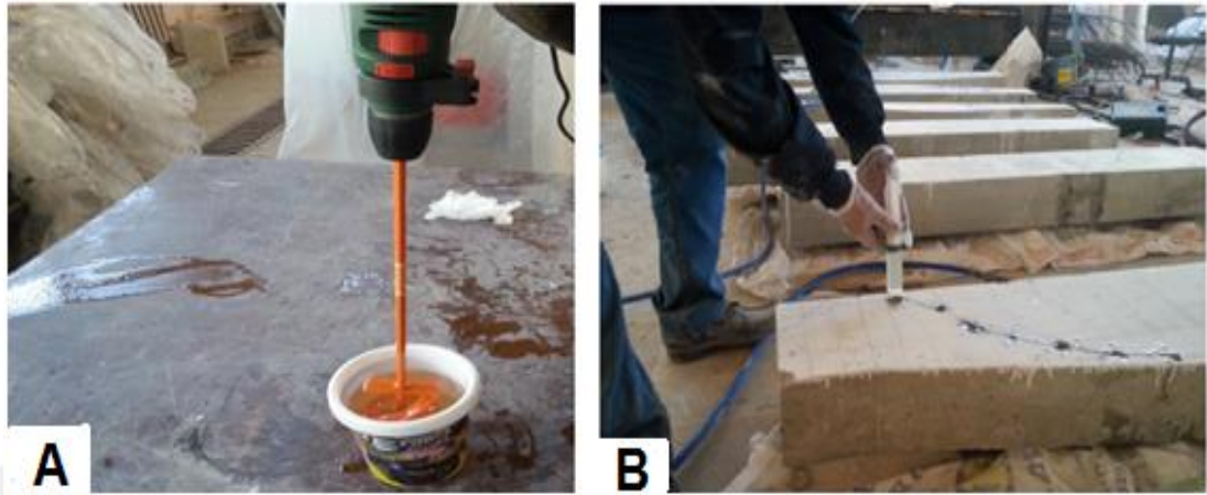
Figure 3.8 (A) Mixing epoxy A+B by using a suitable mixer (b) injection epoxy by gravity.
