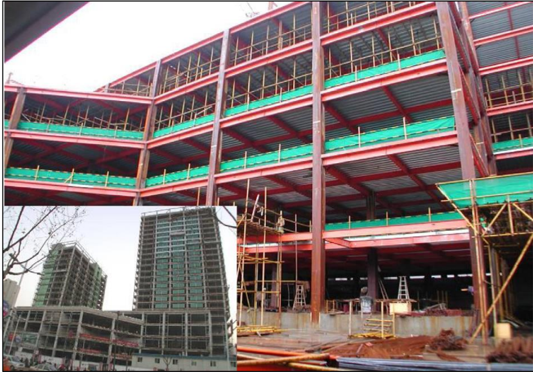
Figure 1.6 Steel-concrete composite column structure (Ruifeng building in Hangzhou - China) (Han et al., 2014)
