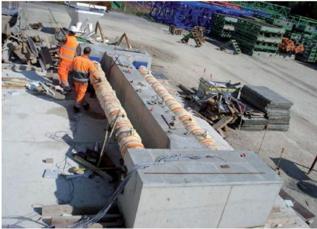
Figure 1.3 Block with restrained shrinkage (I shape beam and steel strut) (French national research program, 2014)
