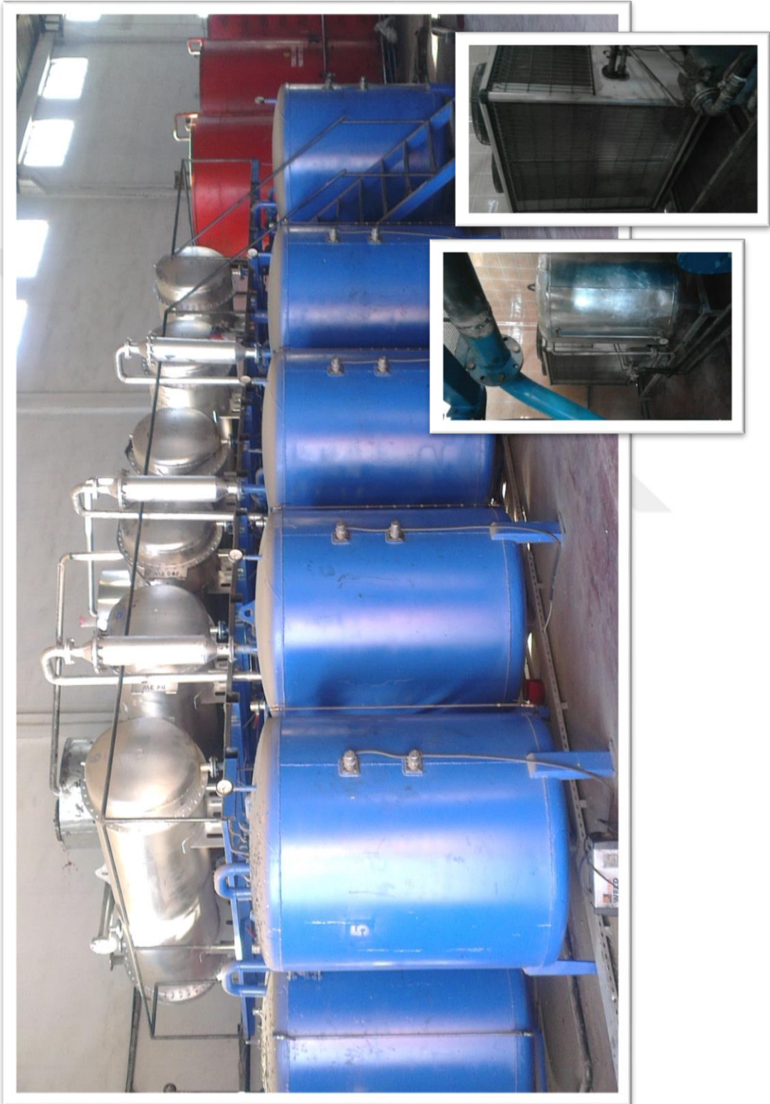
Figure A.1 The lube oil recycling unit
