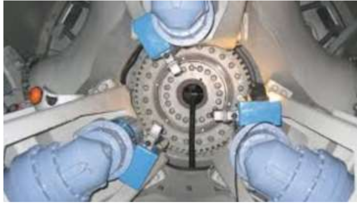
Figure 3.12 Pitch System in the wind turbine [14]
