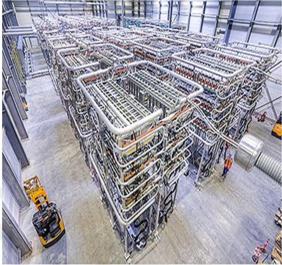
Figure 4.12 Interior view of a converter station HVDC-MMC link [57].
