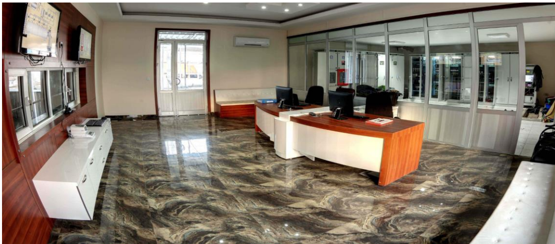
Figure 4.8a Automation and control room of the incineration plant
