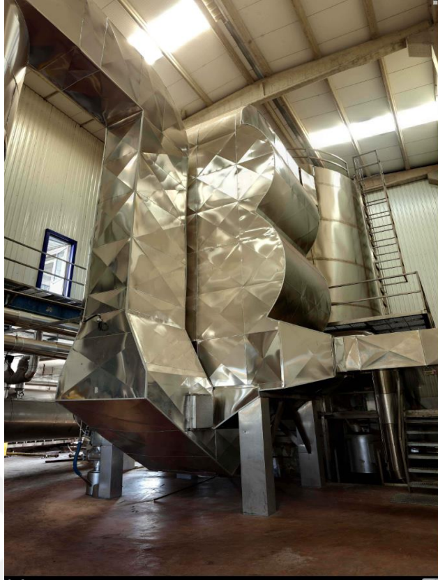
Figure 4.9 Incineration unit with economizer
