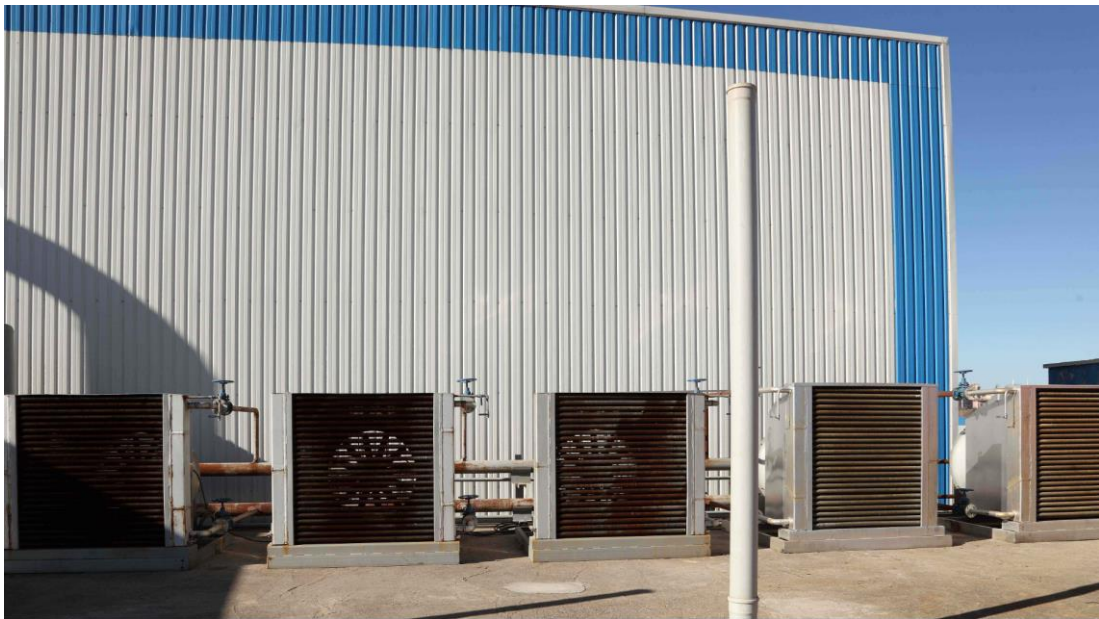
Figure 4.6 Oil heat exchangers
