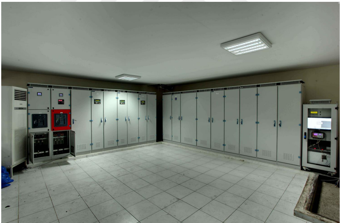
Figure 4.7 Electric room of the incineration plant
