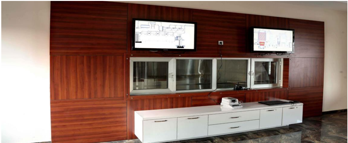
Figure 4.8b Automation screens of the incineration and thermal drying system
