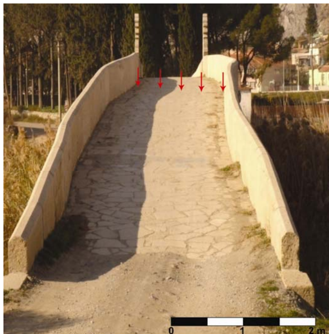
Figure 4.18: Sudden bending on the Ottoman bridge (~50 cm) pointed with red arrows (looking towards northwest).
