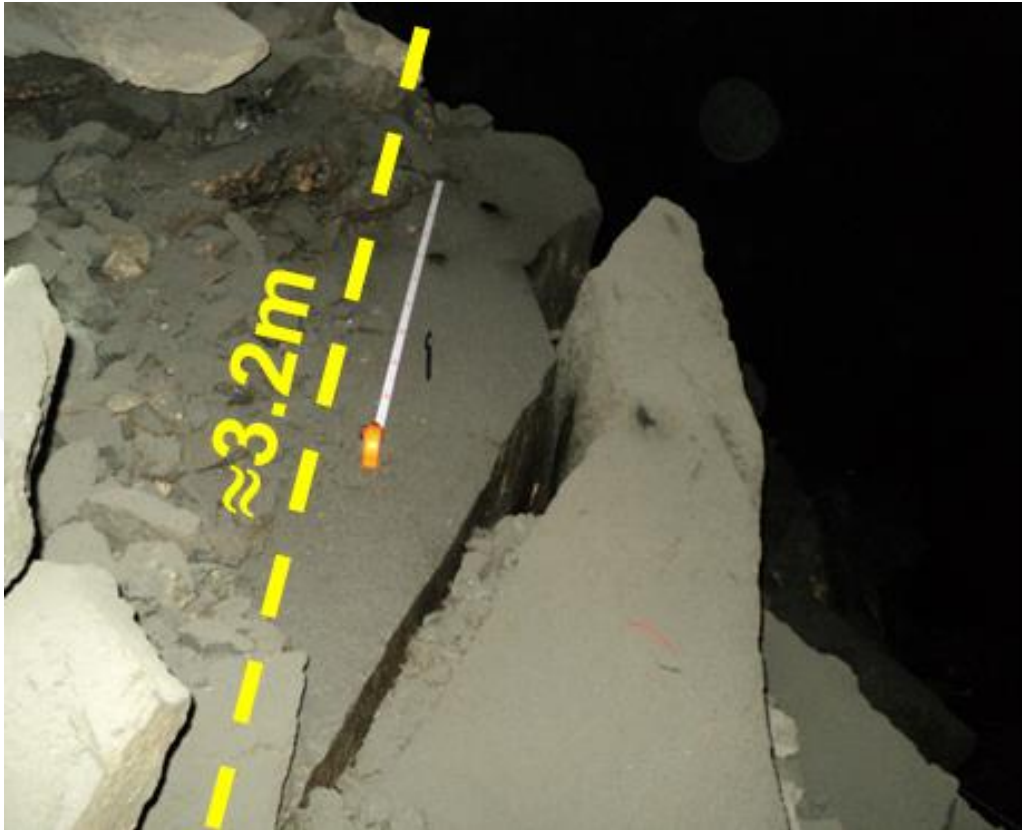
Figure 3.13. Rock falling of blocks from the back of the stope in central ore body at a mining depth of 693 m
