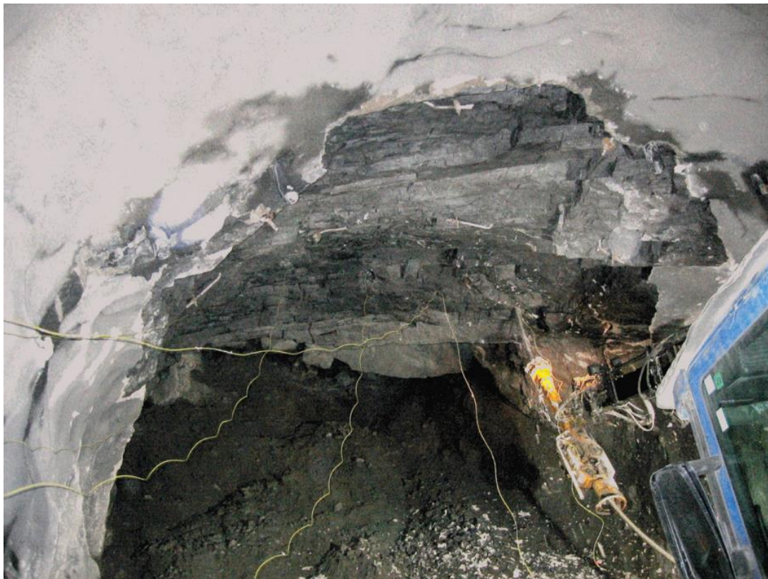
Figure 2.3. Blast-induced spalling close to blast source (Zhang, 2017)
