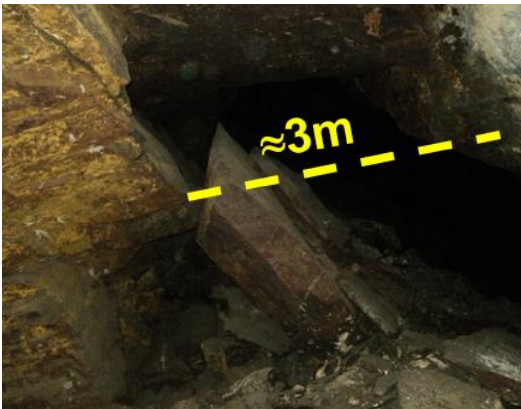
Figure 3.12. Rock falling of blocks from the back of the stope close to post-pillar in central ore body at a mining depth of 693 m
