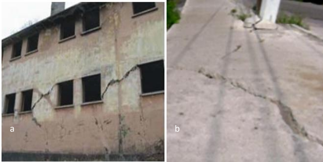
Figure 4. 16 a-Deformations on building (Turer et al. [78]) and b-Deformations on ground (Can et al. [34])
