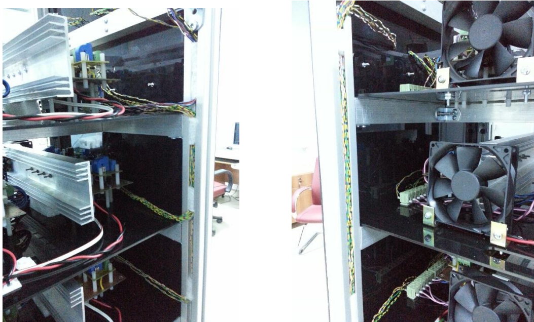
Figure 4.12 Motor drivers cable management and cooling fans (3 shelf)
