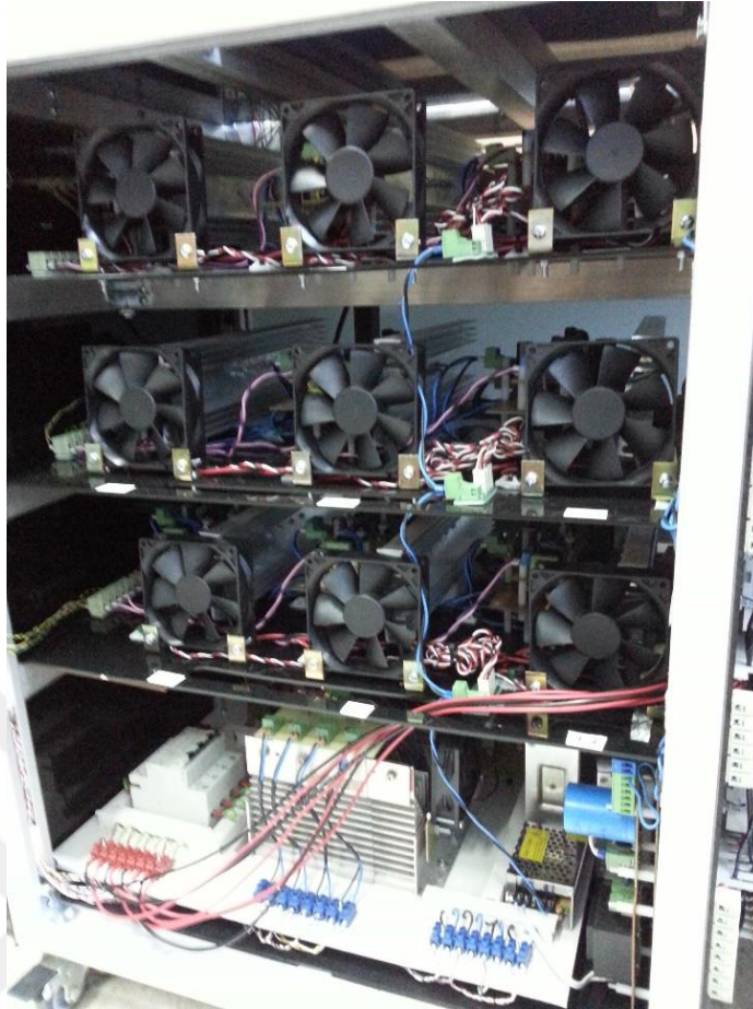
Figure 4.14 Complete system, three shelf H-Bridge driver and one shelf linear driver
