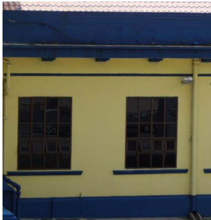
4. The whole window panels as upper image have been changed to glass
