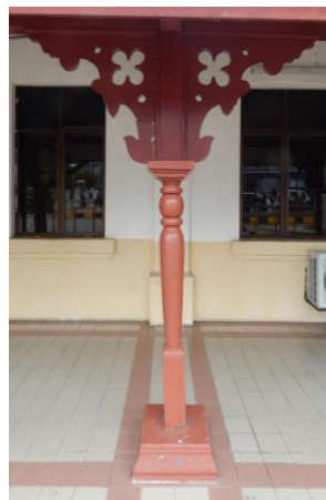
Figure 4.48 Timber column with decorative floral motifs on its spandrels of Seremban station building
