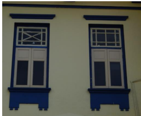
5. The same window panels as upper image but the window panels on louvered parts have been changed to glass
