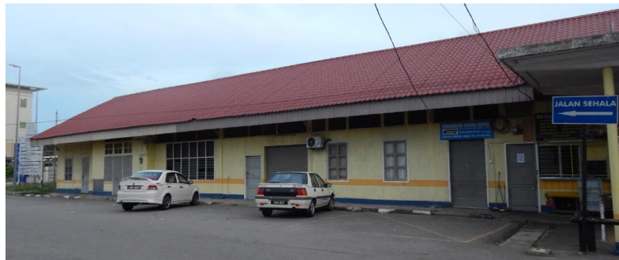
3. Hal of the façade view shows the double panel timber with glass windows, single timber door and the ventilations on the upper window
