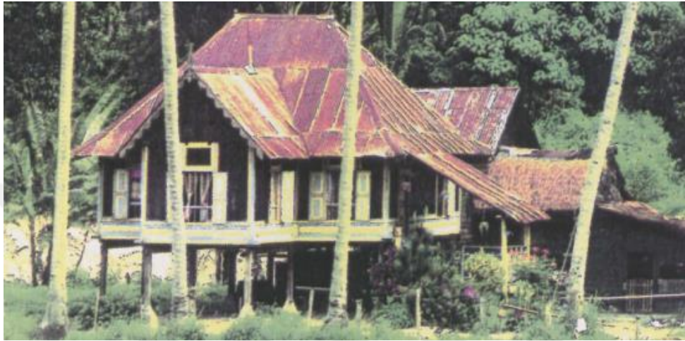
Figure 4.22 The main roof used hipped roof or ‘bumbung limas bungkus’ in a Malay house [30]
