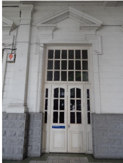
1. Double panels timber glass doors with two fixed timber glass panels on both sides. The upper part lattices are fixed glasses.
