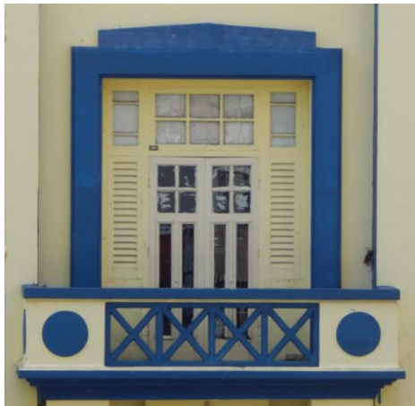
4. The panels still remains but whole timber door has been changed to timber mixed with glass panel doors
