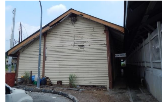
3. The side view of the old station building which was preserved and the new building was built adjacent to it.
