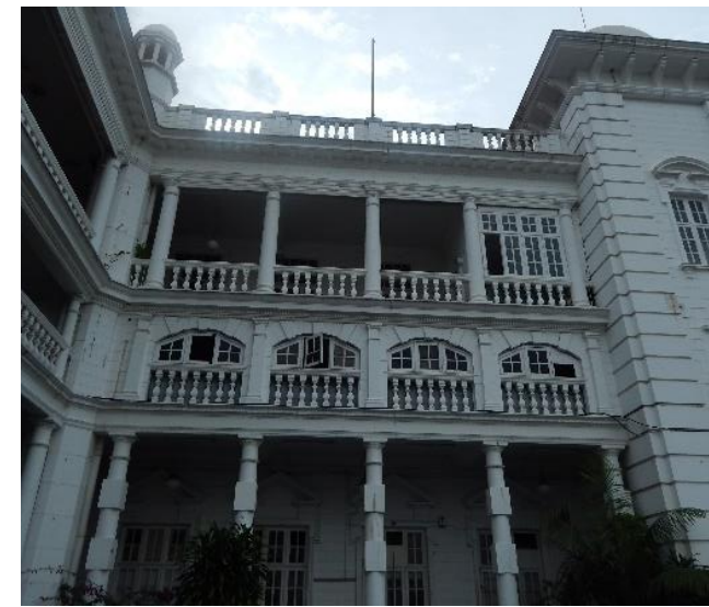
3. The segmental arches later being infill with windows to create more spaces located at the mezzanine floor.
