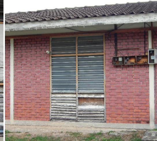
3. Louvered glass panel windows used on both; lower and upper part and timber panels below the windows.
