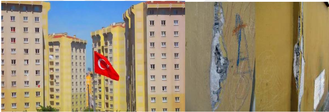
Figure 3.19 TOKI social houses in Ayazma-Tepeusru and the cracking wall photographed by the users (Source: IMO, 2009)
