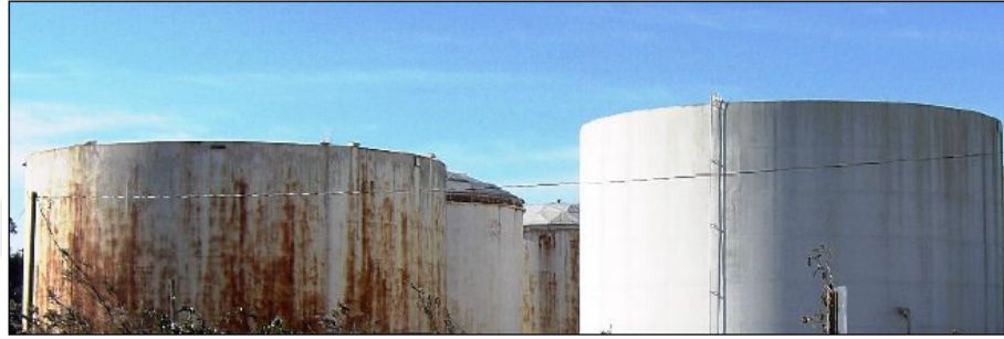
Şekil-2.12 Silindirik tanklarda ve kapalı kaplarda akustik emisyon ile korozyonun incelenmesi ( http://www.techcorr.com/acoustic-emission-testing.php & http://www.idinspections.com/wp-content/uploads/Acoustic-Emission-Inspection-of-Petroleum-Tanks-and-Piping-May-2016.pdf )
