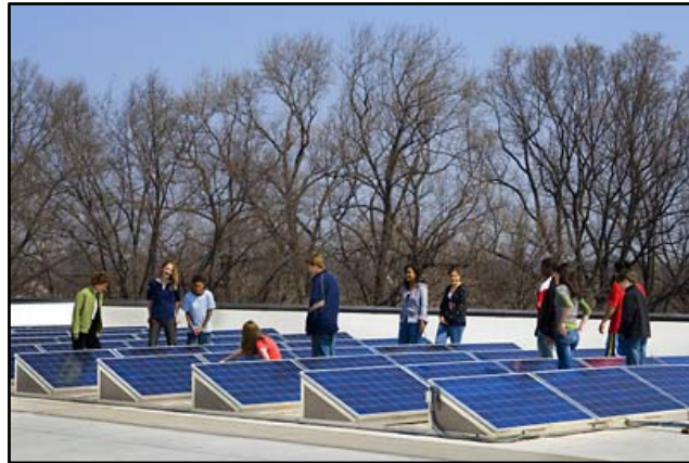
Figure 3.33. PV panel integration on rooftop [65]
