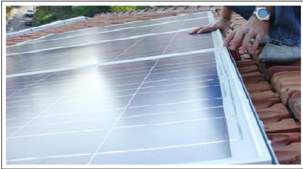
Figure 4.31. A photovoltaic panel on the roof [60]
