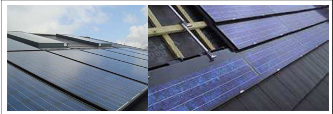
Figure 4.33. Rooftop sidings with mono and poly crystalline photovoltaic panels [60]
