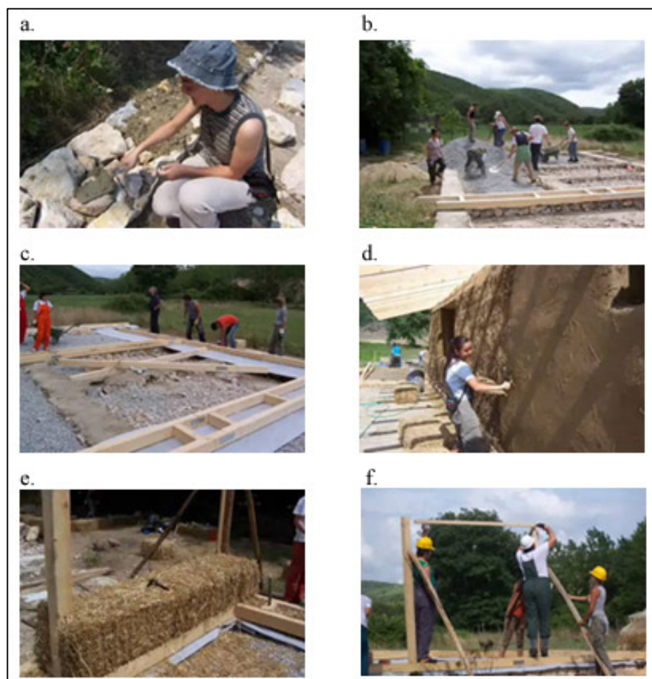
Figure 4.16. Application of straw bale, a. the basic construction of stone, b. preparation of the basic top frame, c. basic surface water insulation, d. plaster over straw, e. straw bale placement, f. gaps in doors and windows [42]
