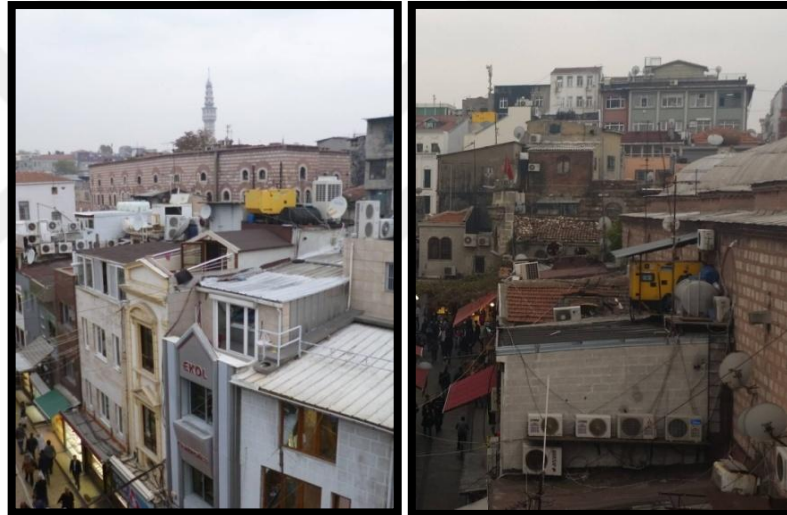
Figure 2.92. and Figure 2.93. Generator on rooftops [13]
