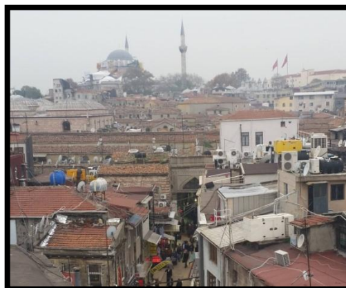
Figure 2.94. Generator on rooftops [13]
