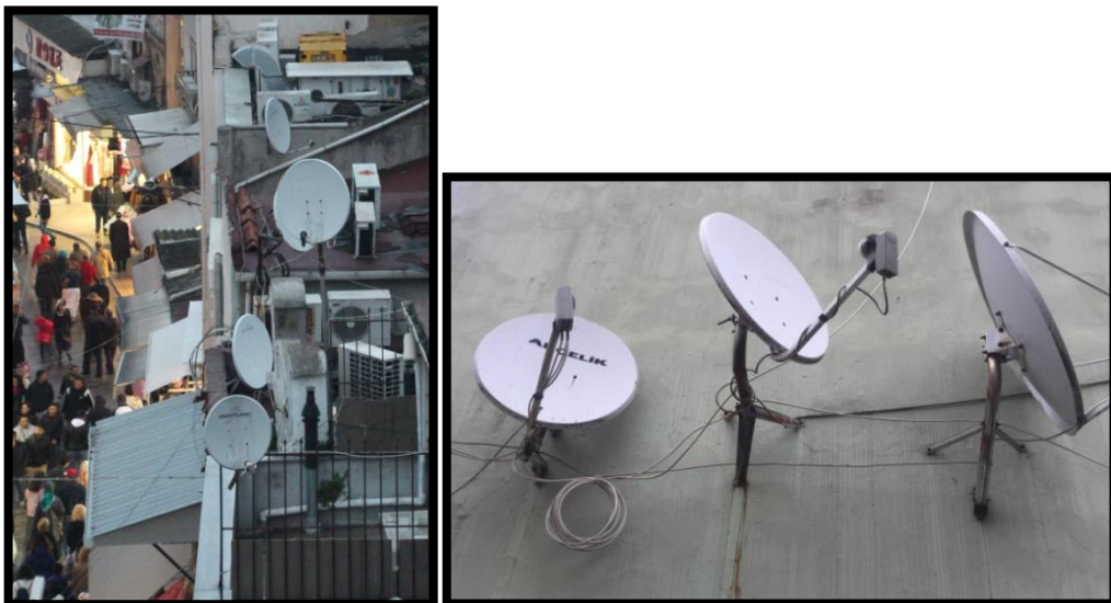
Figure 2.89. and Figure 2.90. Satellite dish detail views [13]
