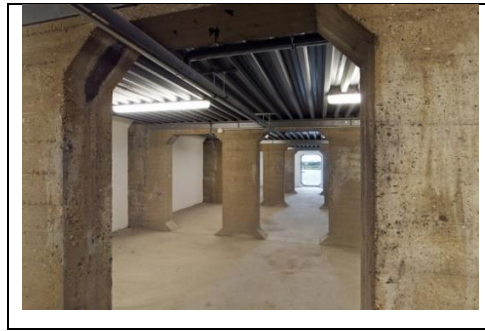
Figure 4.68. The inside of the Kraaspoor showing the remaining wall structure in the corridor used in the new function as fire-escape route [61]
