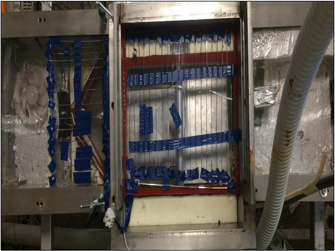
Figure 5.2. Complete test section for the cylindrical condenser
