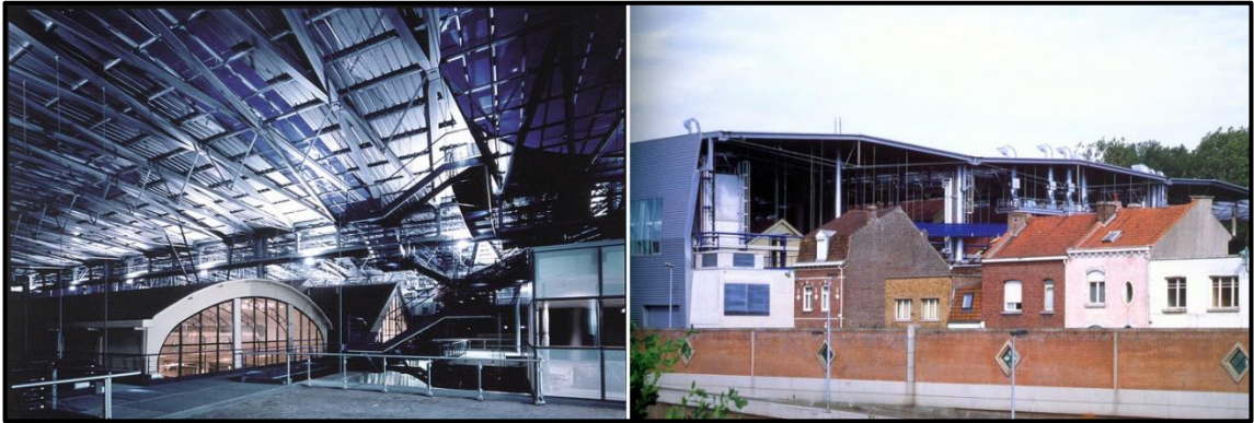
Figure 4.18. Steel roof installed over the existing building, Le Fresnoy Art Center, Bernard Tschumi Architects, 1997 [205]
