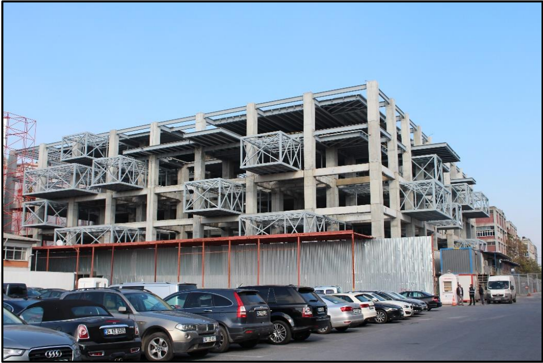
Figure 4.131. Photo of ongoing construction, İstanbul Museum of Painting and Sculpture, Emre Arolat Architecture, 2015 (Photo by author)
