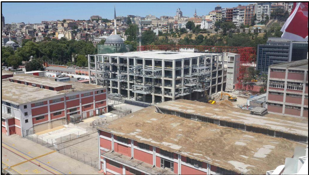
Figure 4.132. Photo of ongoing construction, İstanbul Museum of Painting and Sculpture, Emre Arolat Architecture, 2015 (Photo by author)
