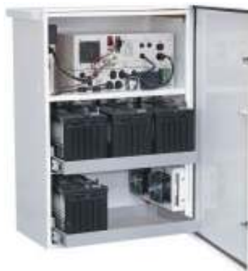
Figure 3.26. Sample outdoor UPS system
